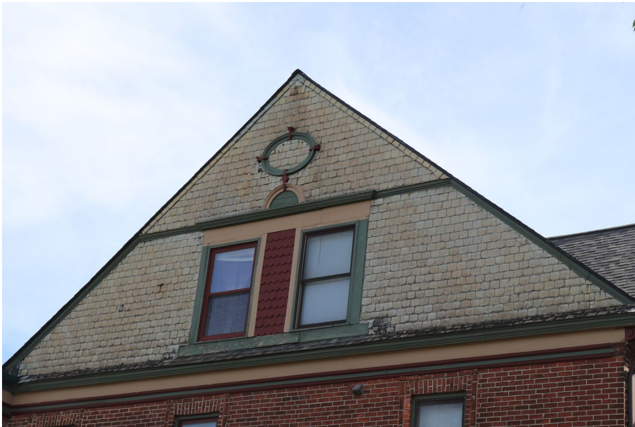
South-West facing gable end, facing the Brush Street side, shows areas of deterioration, rusted nails, slipping tiles, as well as a few areas of replaced tiles (see detailed photos on next page)
