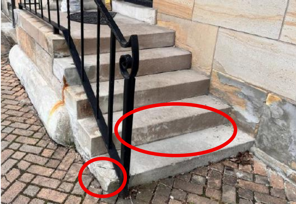
Both photos above, from applicant materials, show deterioration and insensitive repairs on the side porch's cap and steps.
