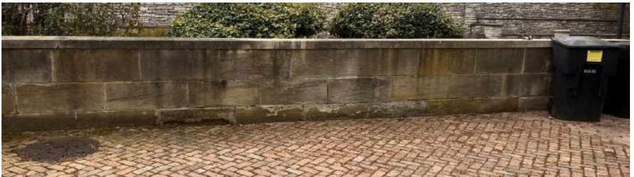
Photo from applicant materials of service court wall to be rebuilt with in-kind materials and with the same dimensions as the existing wall. (Dimensions of existing and proposed need to be submitted to staff.) Staining and deterioration is evident.
