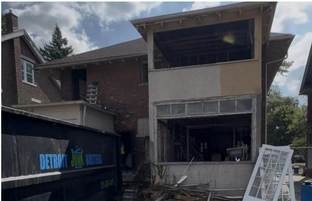
Rear, showing unapproved demolition of the two-story sunroom wing in progress. Photo by applicant
