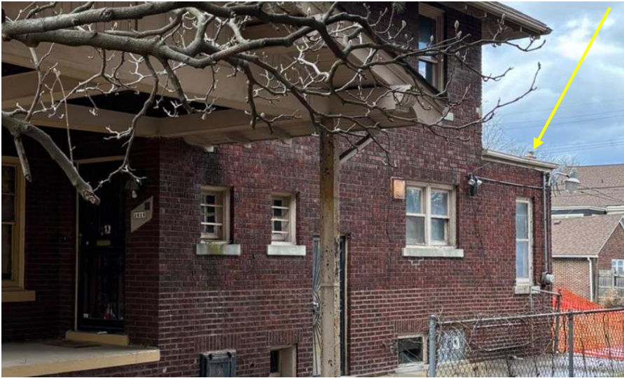
Rear, one-story wing, showing current brick veneer cladding (yellow arrow). Photo by applicant.
