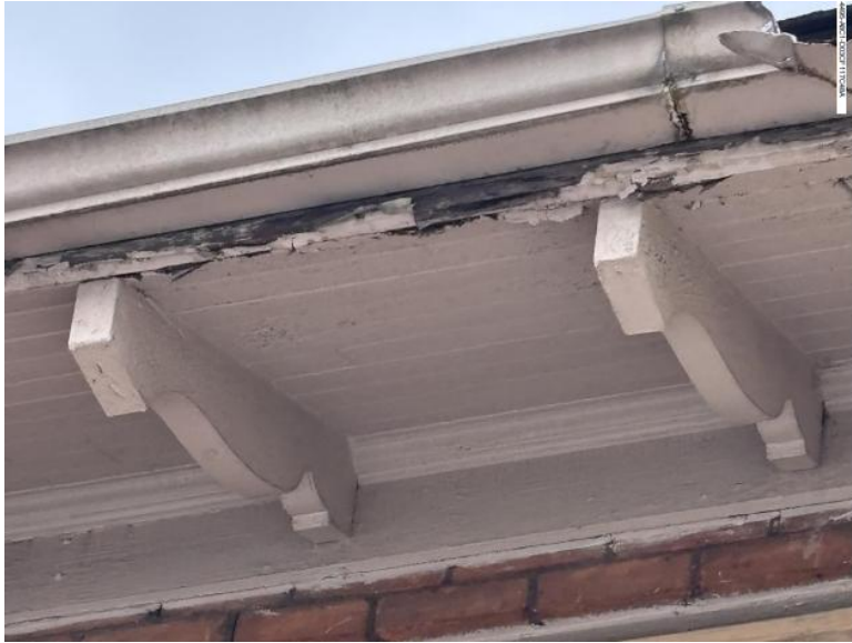
Photo detailing conditions at the main roof's eaves/soffit/fascia. Note that a similar detail photo of the eaves/soffit/fascia of the former rear 2-story sunroom wing do not exist as the element was demolished without such documentation. Photo by applicant
