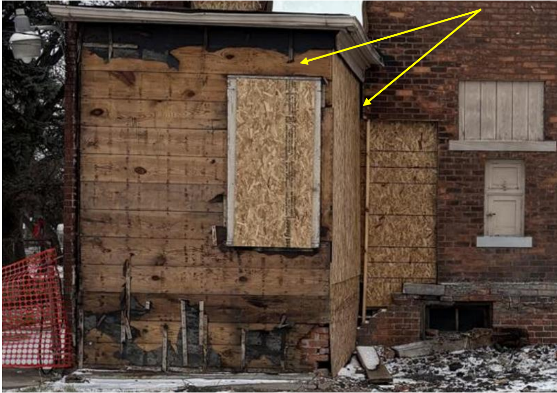
Rear, one-story wing, showing current conditions after stucco was removed from rear and west walls without HDC approval (yellow arrows). Photo by applicant.
