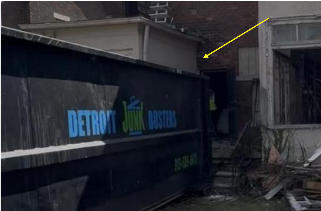
Rear, one-story wing, showing stucco cladding which was removed from west wall without HDC approval (yellow arrow). Photo by applicant.
