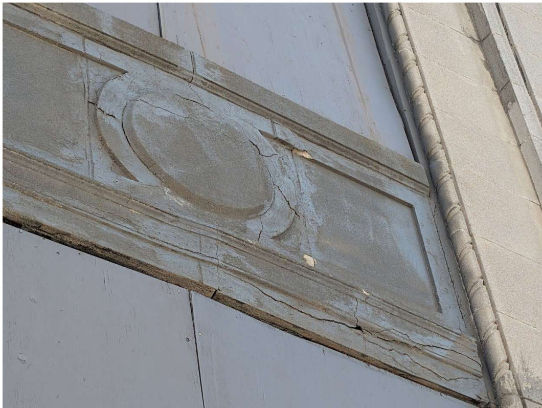
Detail photo of spandrel panel showing multiple areas of failure. Staff photo, April 23, 2026.
