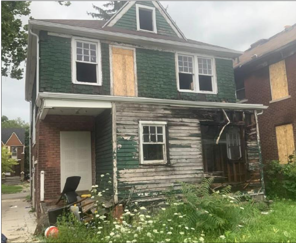
Applicant photo. With exception of the deteriorated section of the wall, the historic age wood siding on the remaining walls appeared to be intact and in repairable condition.
