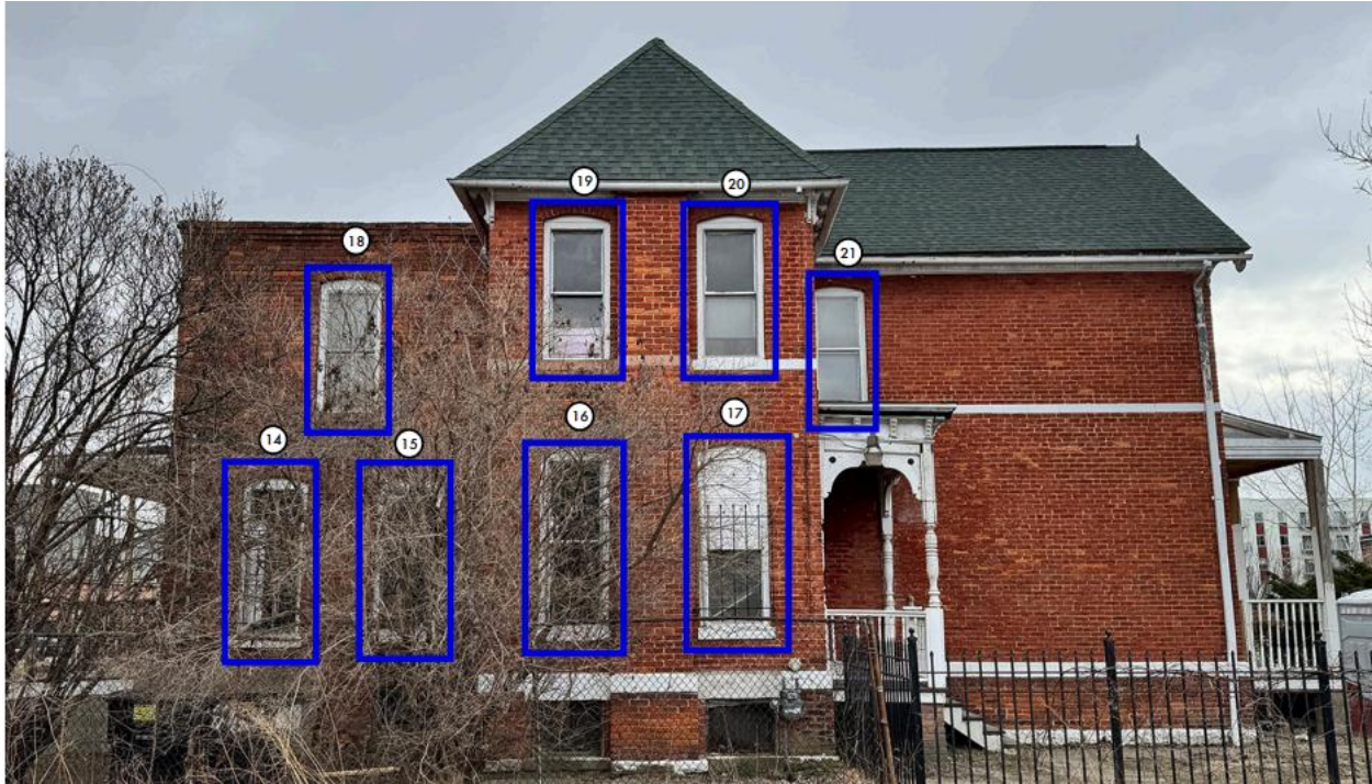
264 Watson, east side wall, by applicant. Windows proposed for removal outlined in blue
