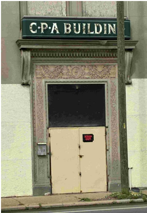
Sign proposed for repair/rehabilitation. Located at east façade, first story. Photo by staff, 3/26/2026
