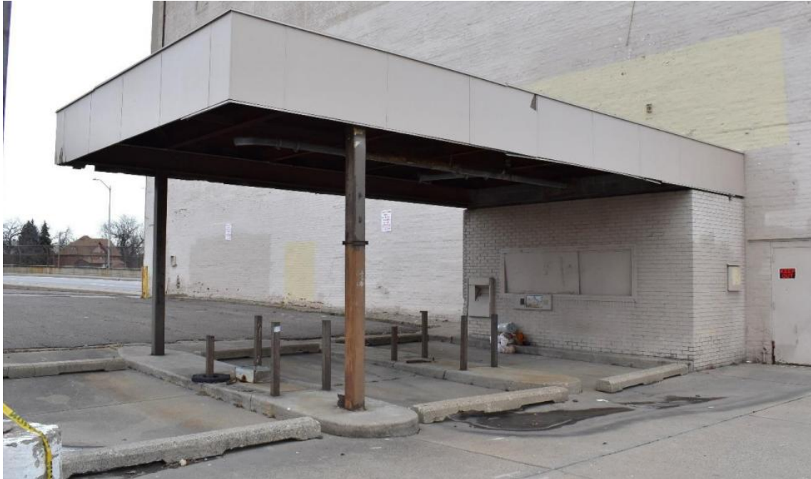
Current appearance. Photo by HDAB, 2025. Facing northeast towards west façade drive through canopy which was installed in 1977
