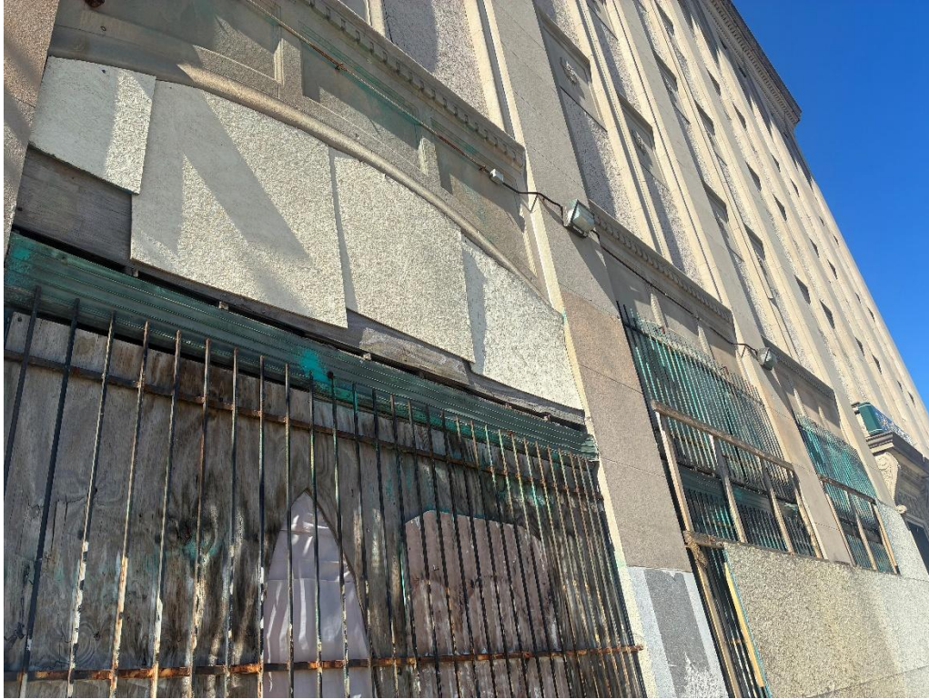
Current appearance. Photo by staff on 03/26/2026. Facing southwest, showing current storefronts covered with plywood panels
