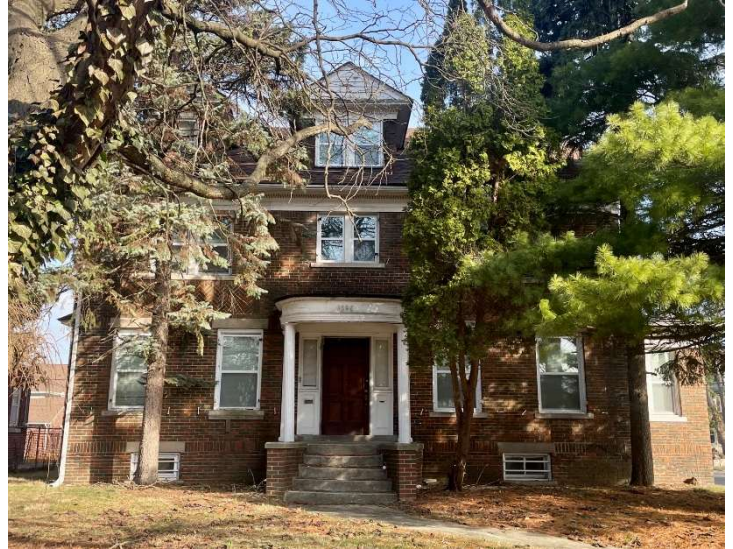
Staff photo, 03/24/2026, showing vinyl windows installed without approval
