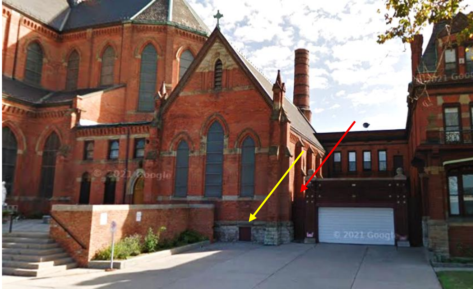
Yellow arrow indicates west elevation opening proposed for enclosure with masonry infill. Red arrow points to south elevation, where openings are proposed for infill with louvered vents (with brickmould to match the existing). One below-grade opening at this location is proposed for masonry infill. The garage blocks the south facade openings from view from the right-of-way. Google Streetview, 2009
