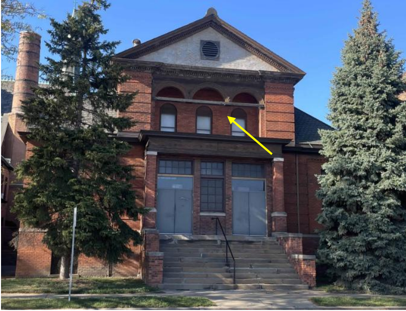
Parish hall, current appearance. Photo by applicant. Arrow to indicate location of proposed new columns to replace missing historic elements
