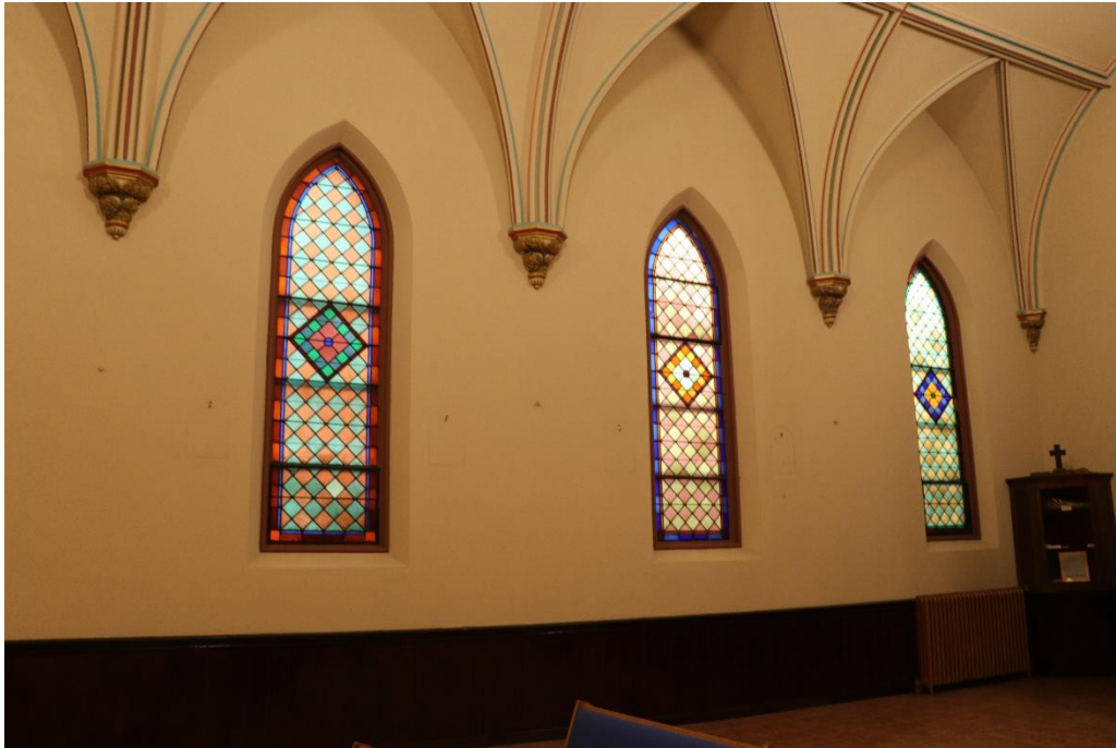
South wall of the Chapel has pointed-arch windows. Note low wood wainscoting and lack of trim at wall around window openings. Photo by staff
