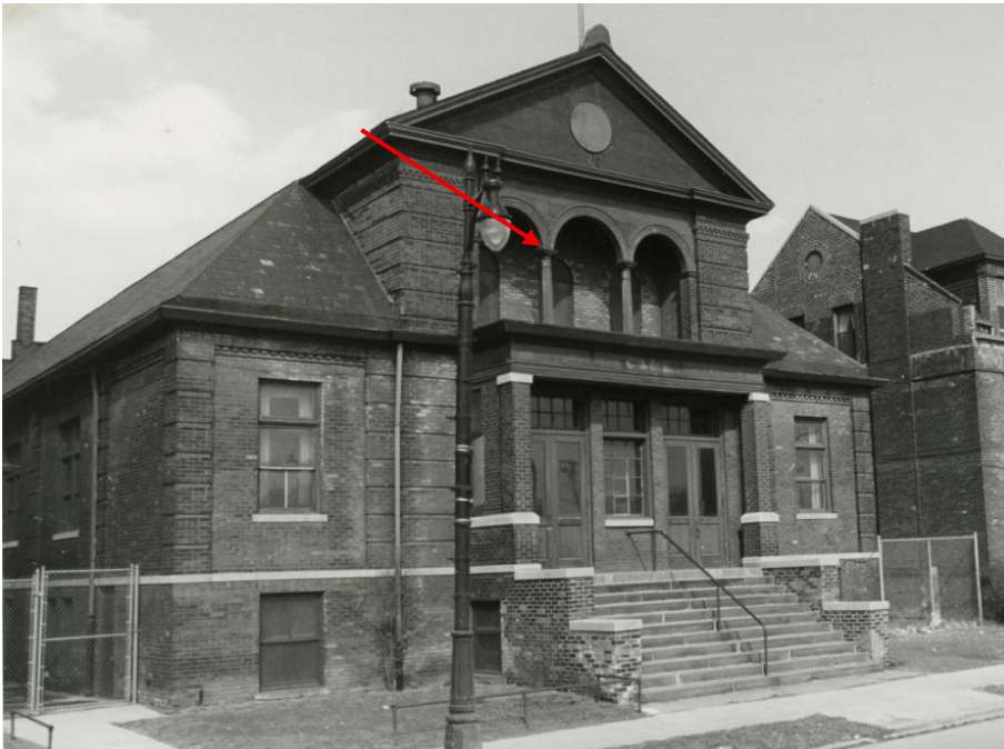
Photo from the NRHP nomination, showing the historic columns at the second story porch which are currently missing and proposed for replication with new urethane columns (red arrow)
