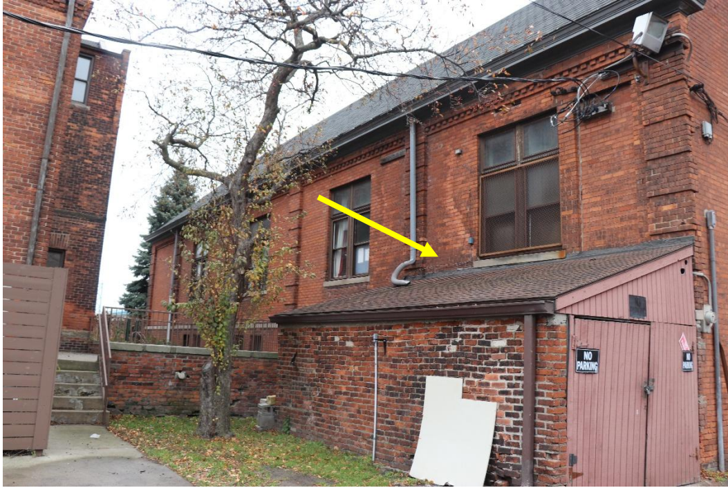
The shed addition at northeast corner proposed for removal (yellow arrow). Staff does not find this addition to be historic or character defining and does not object to its removal. (Staff photo, November 2025)
