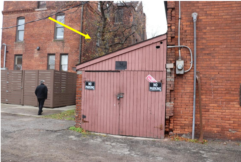
The shed addition at northeast corner proposed for removal (yellow arrow). Staff does not find this addition to be historic or character defining and does not object to its removal. (Staff photo, November 2025)
