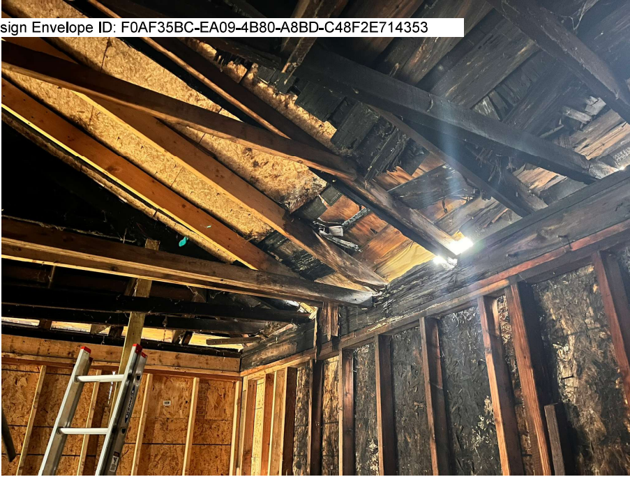
IMAGE 16: PLYWOOD TO SECURE PROPERTY AND STRUCTURE - WATER DAMAGE ON SOME PLYWOOD ELEMENTS DUE TO HOLE IN ROOF - MULTIPLE UNCONNECTED SUPPORT ELEMENTS
