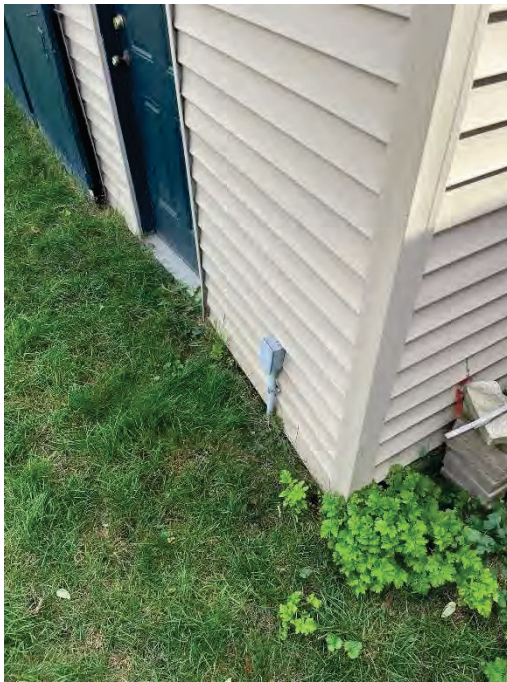
Section of wall severely out of square – not supported by foundation
