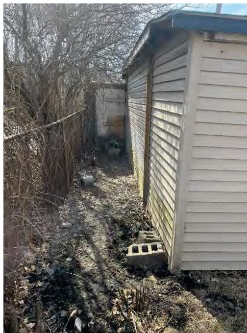
Walls out of plumb, missing fascia, rodent den (at CMU blocks)
