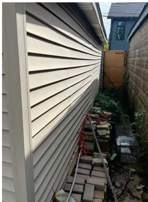
Buckling evident in exterior wall – west side
