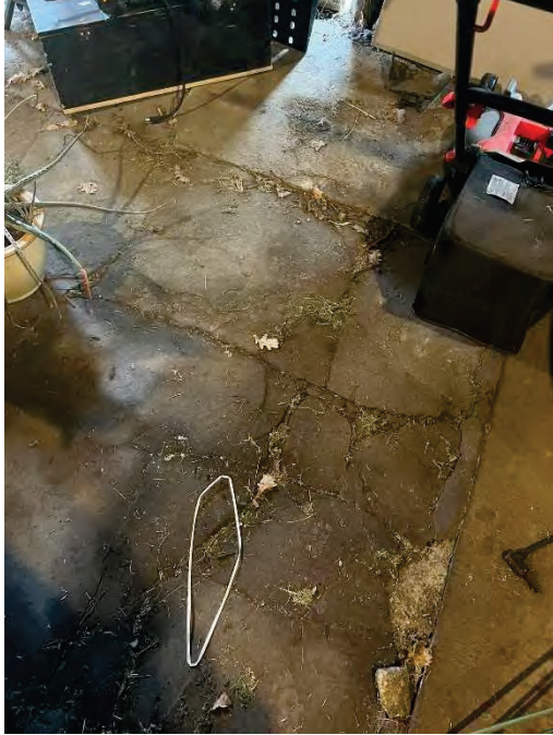
Interior concrete slab deterioration
