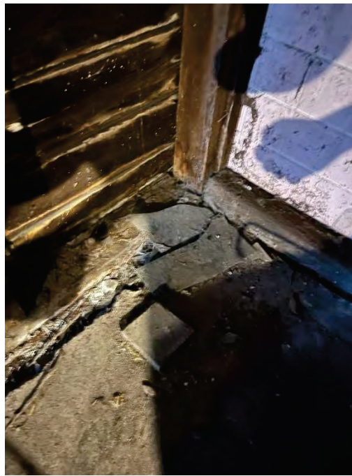
Deterioration of slab and sill
