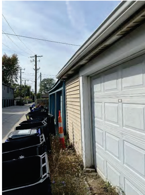
Exterior wall out of plumb
