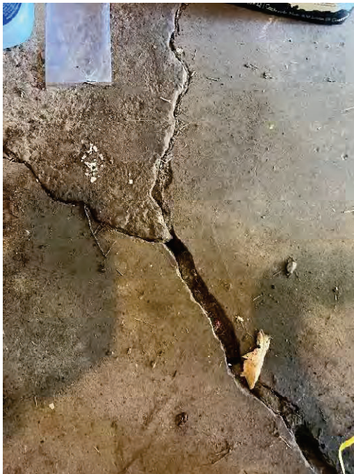
Deterioration of slab
