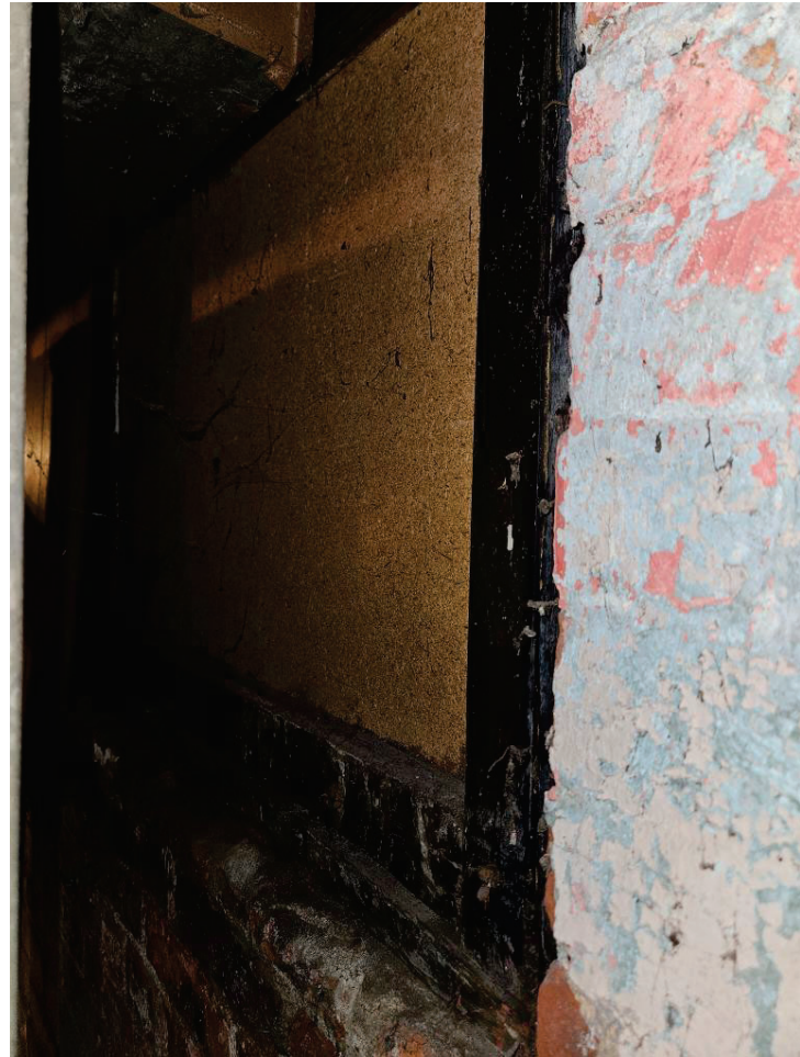
Unit 101 (basement) Exterior – Interior Window is missing and behind the HVAC
