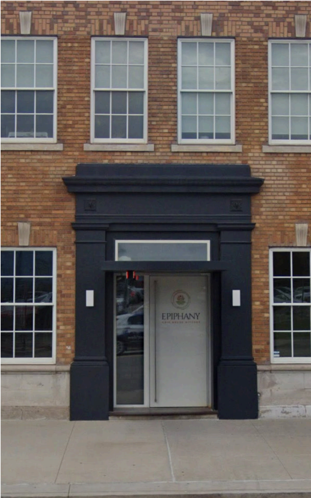
LIMETSTONE PORTAL AND CANOPY, CURRENT CONDITION
