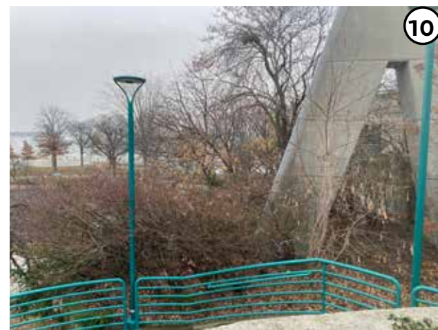
Shrubs vastly overgrown, prune back significantly to reduce size
