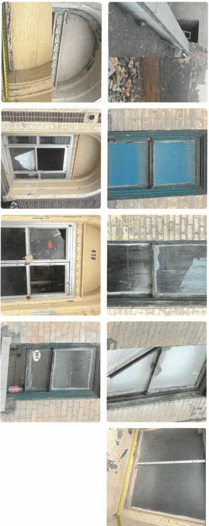
Existing conditions documentation revealed severe deterioration of original wood window assemblies beyond feasible repair.
