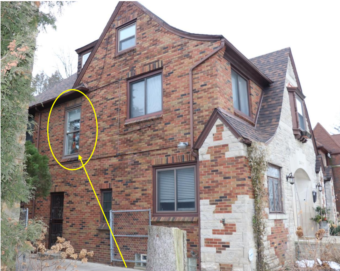
Photo by HDC staff, February 2020, Window proposed for replacement
