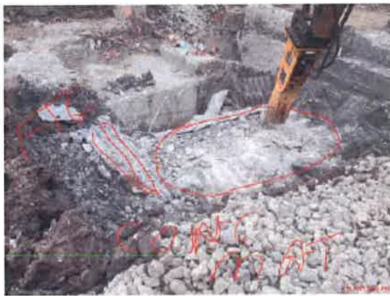
Pictures of some of the unexpected underground obstructions
