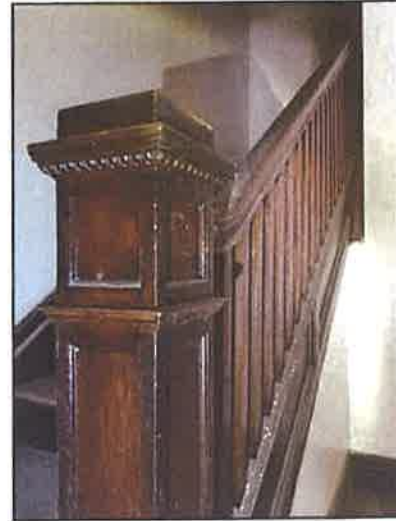
Newel posts and bannisters like these ca. 1910 will be refurbished where applicable
