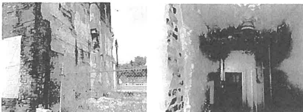
Existing building located at 1314 Gratiot Avenue (left) and the interior of 1325-1337 Maple Street (right)
