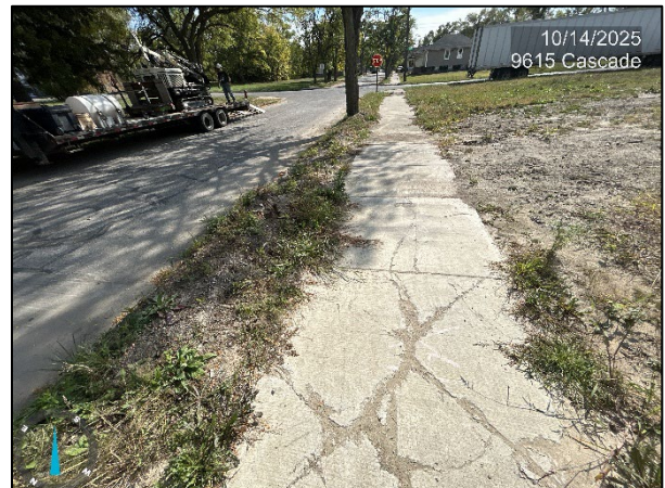
Photo 6: Viewing broken sidewalk in front of the Site prior to drilling
