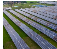
The Solar Park at O'Shea, on Detroit's West Side, is a 2.44 Megawatt solar installation.
