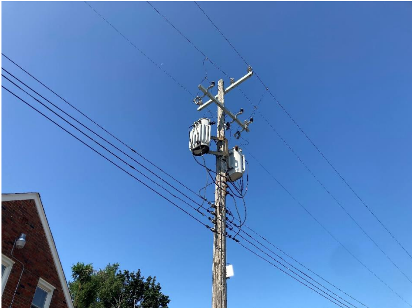
Pole-mounted transformers located along the southern boundary at 19505 Grand River Avenue
