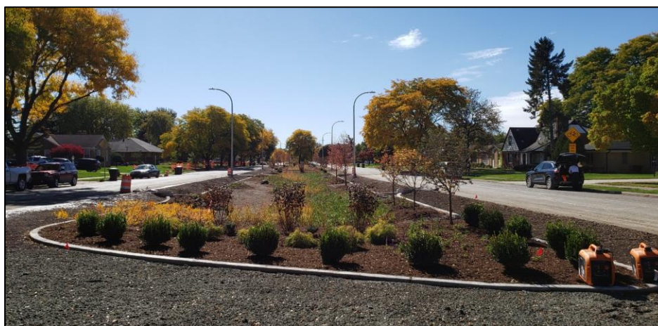
Figure 1 Oakman Boulevard Green Stormwater Infrastructure
