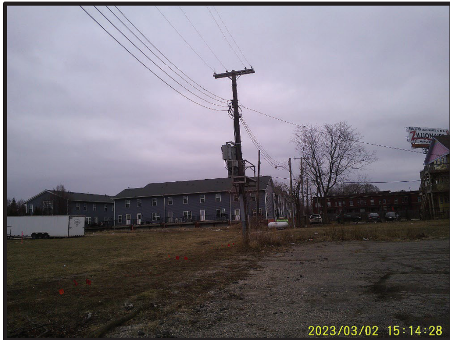
Photo 12. View of pole mounted transformer within the electrical transmission utility easement that transects the central portion of the Subject Property.
