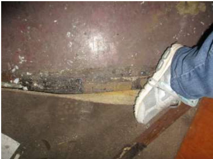
Photo 8. A view of the asbestos-containing 9"x9" floor tile beneath carpet
