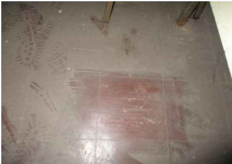
Photo 9. A view of the asbestos-containing 9"x9" floor tile
