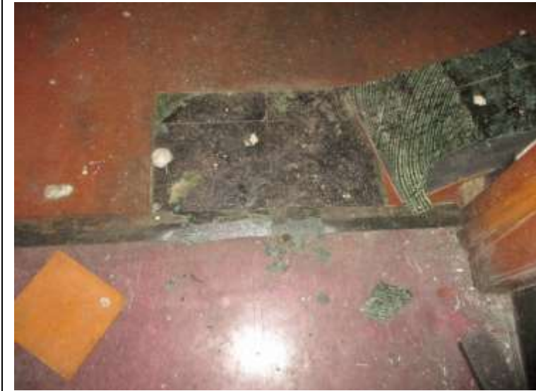
Photo 10. A view of the asbestos-containing 9"x9" green floor tile beneath carpet
