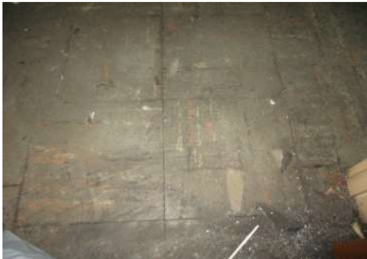
Photo 3. A view of the asbestos-containing 9"x9" floor tile
