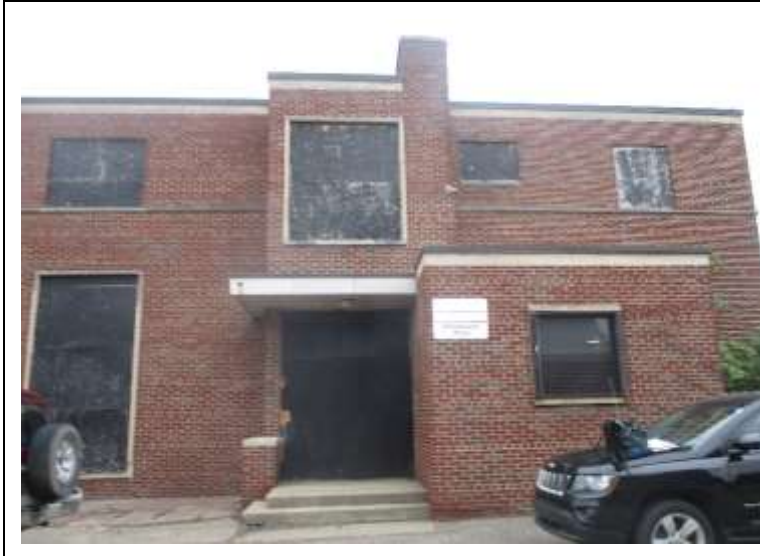
Photo 4. A view of the asbestos-containing caulk on overhang
