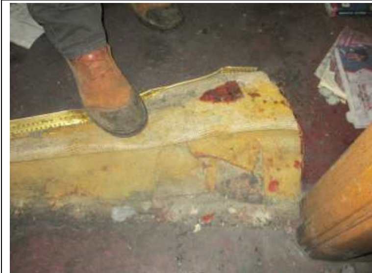
Photo 11. A view of the asbestos-containing 9"x9" red floor tile beneath carpet+
