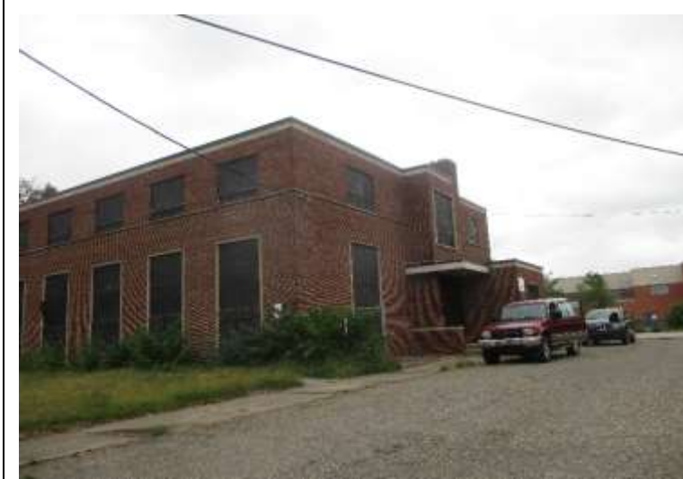
Photo 5. A view of the asbestos-containing caulk on overhang
