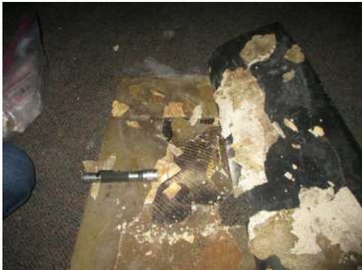
Photo 2. A view of the asbestos-containing floor tile beneath carpet
