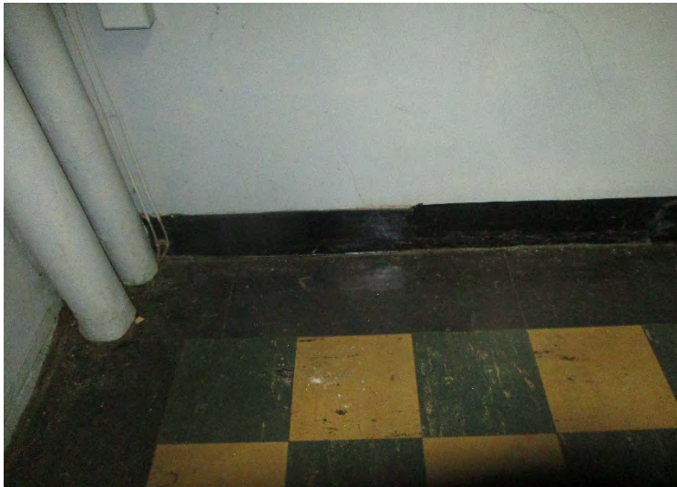
Photo 23. A view of asbestos-containing cove-base in classroom 102
