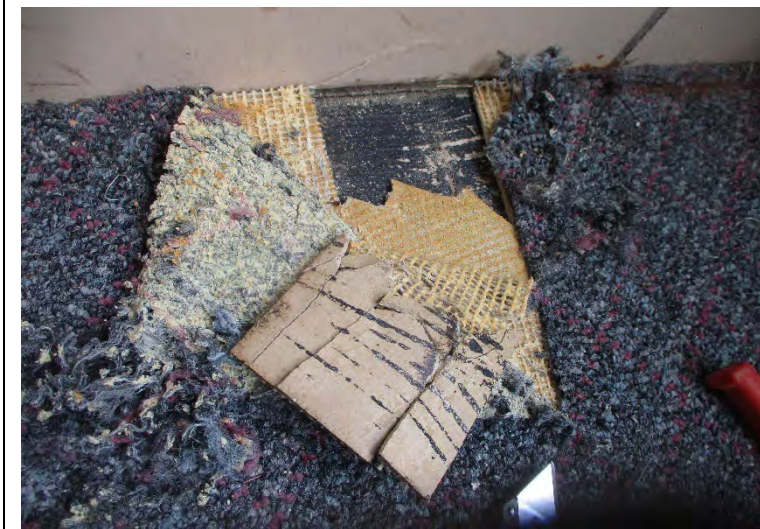
Photo 6. A view of asbestos-containing floor tile beneath carpet in the 5959 Whittier office
