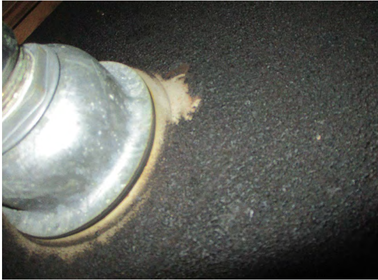
Photo 7. A view of asbestos-containing sink undercoating in the kitchen of 5959 Whittier.
