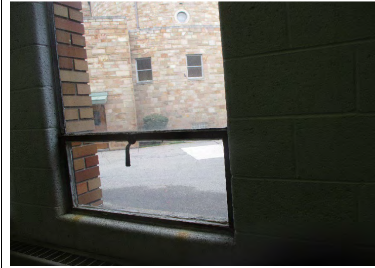
Photo 31. A view of asbestos-containing window glaze
