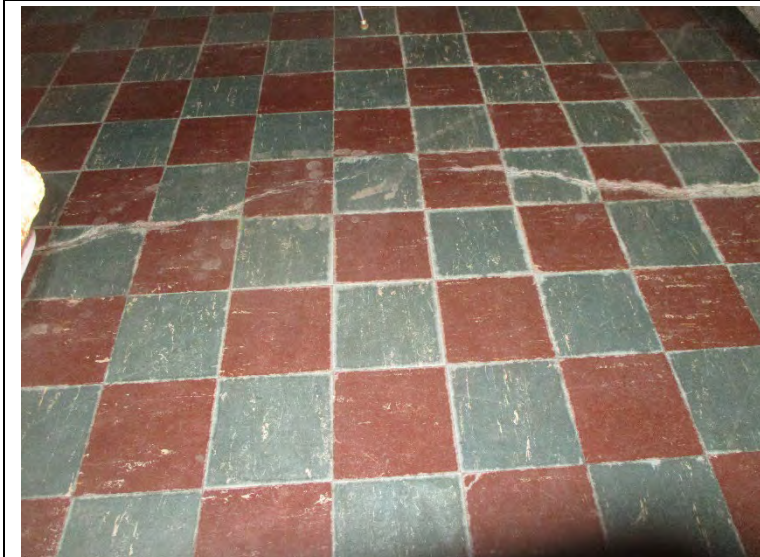
Photo 14. A view of asbestos-containing 9"x9" floor tile in the Cafeteria in the 5970 Audubon building
