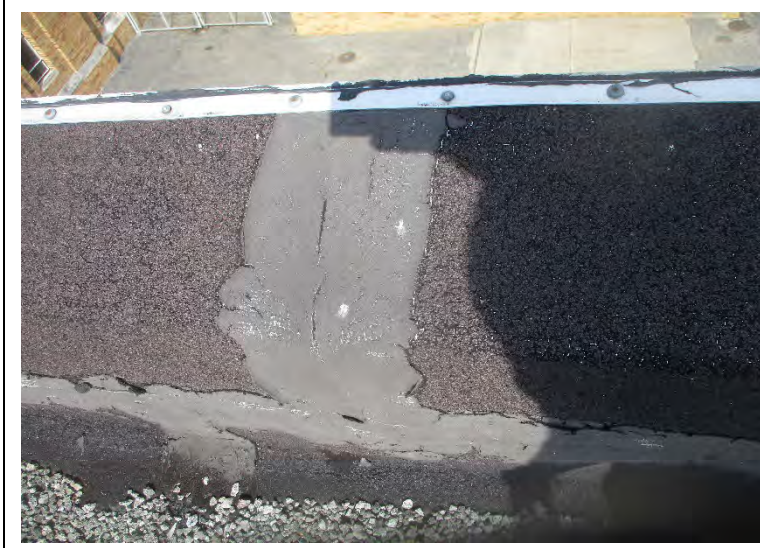
Photo 13. A view of asbestos-containing flashing
