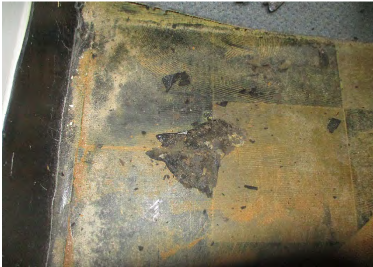
Photo 26. A view of asbestos-containing 9"x9" floor tile beneath carpet in room 105
