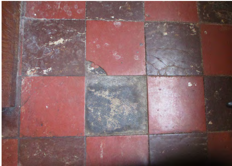
Photo 17. A view of asbestos-containing 9"x9" floor tile in the kitchen in the 5970 Audubon building
