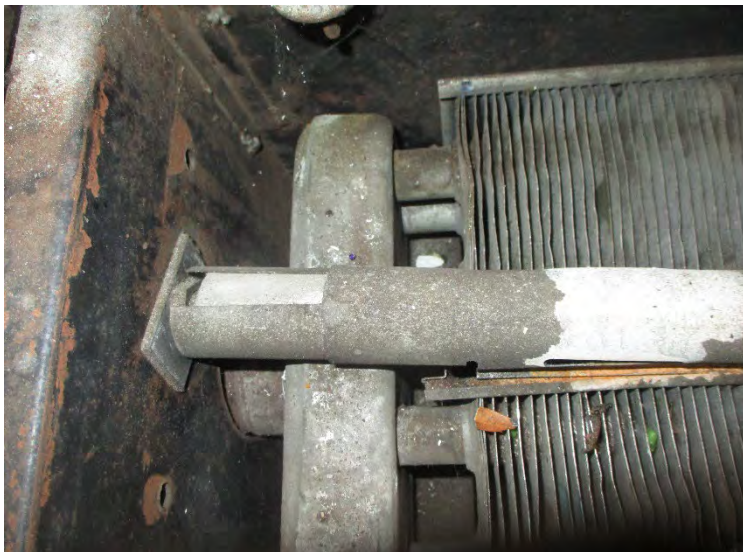
Photo 33. A view of asbestos-containing radiator spacer
