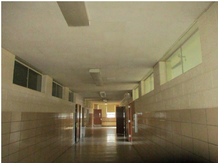
Photo 8. A view of asbestos-containing window caulk on 1 st and 2 nd floor hallway windows (between hallway and classrooms)
