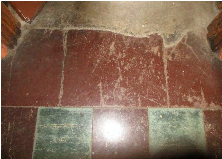
Photo 18. A view of asbestos-containing 16"x18" border floor tile in the kitchen in the 5970 Audubon building
