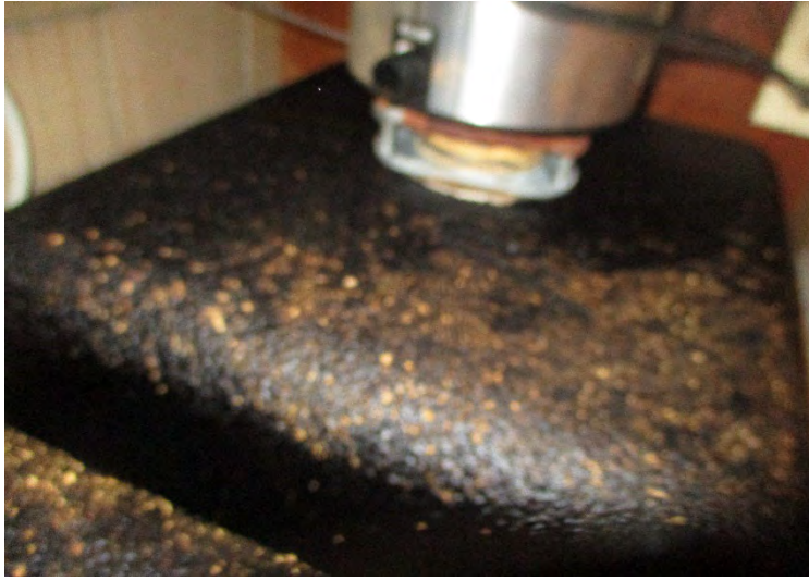
Photo 19. A view of asbestos-containing sink undercoating
