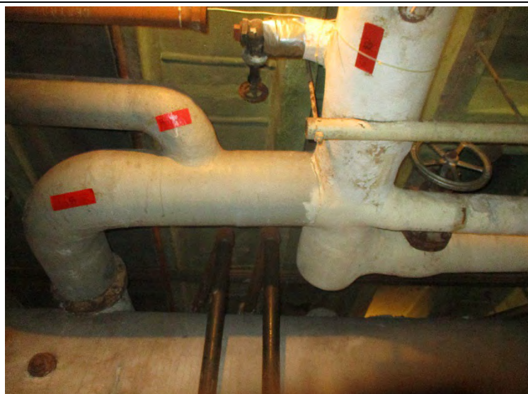
Photo 12. A view of asbestos-containing pipe wrap and mud-joint insulation in the 5970 Audubon building
