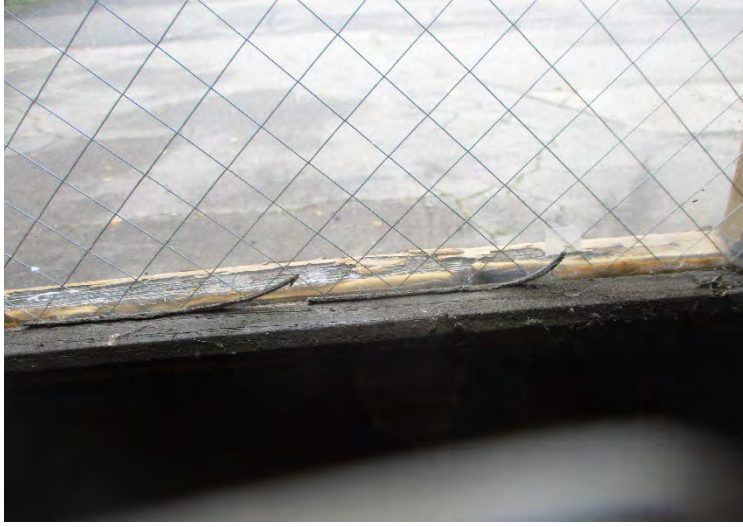
Photo 28. A view of asbestos-containing window glaze on the west stairway door
