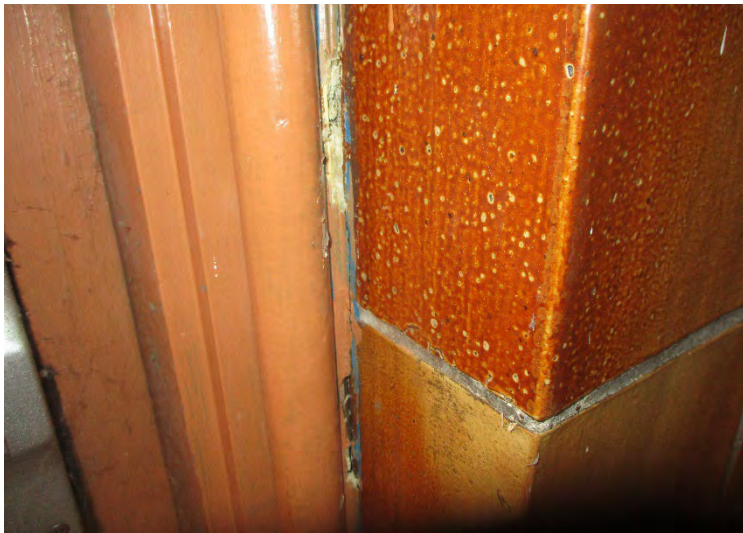
Photo 27. A view of asbestos-containing interior Gym door caulk
