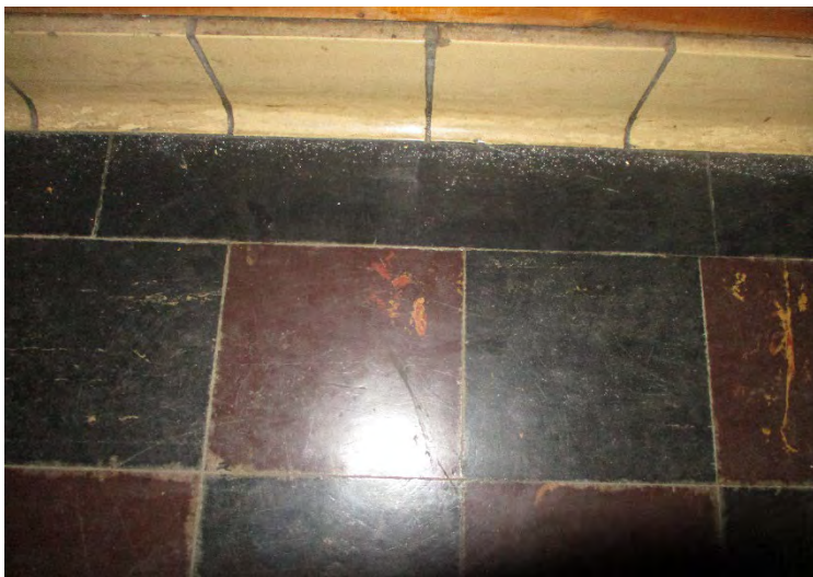
Photo 21. A view of asbestos-containing 12"x4" floor tile border in the hallway
