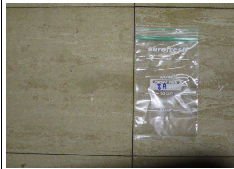
Photo 4. A view of asbestos-containing 9"x9" Floor tile in the 1 st and 2 nd floor classrooms in 5959 Whittier building
