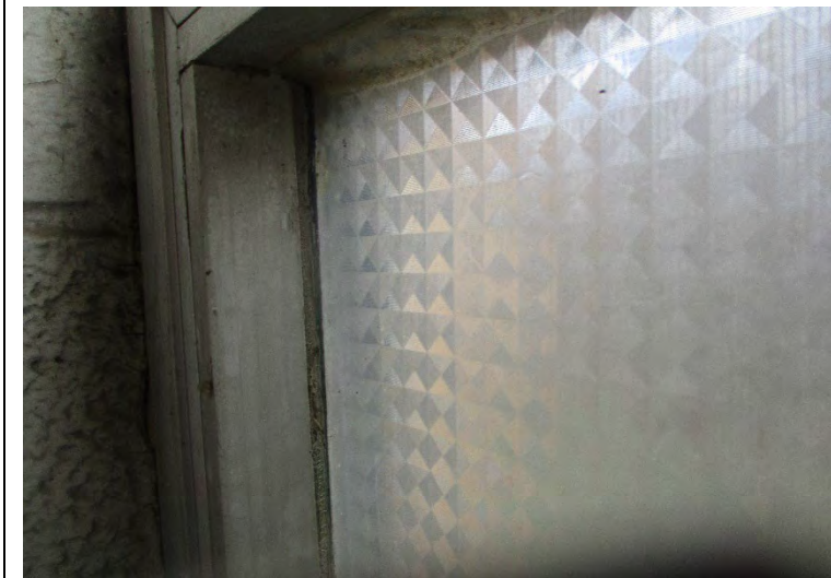
Photo 5. A view of asbestos-containing window glaze
