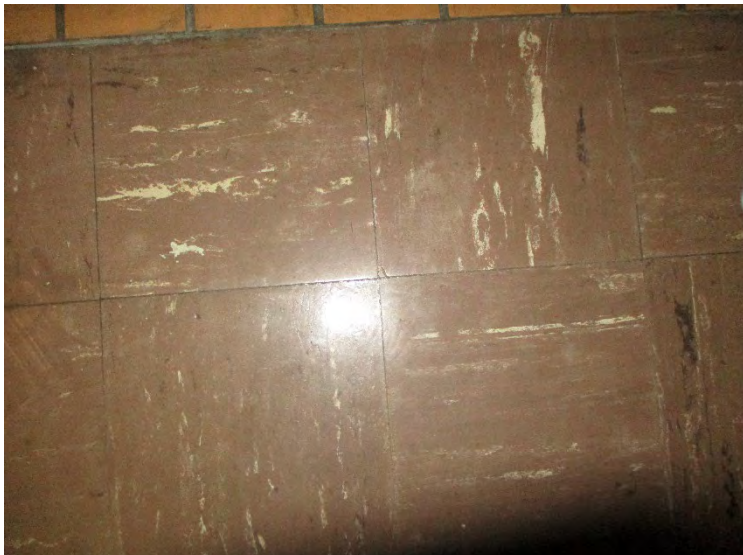
Photo 29. A view of asbestos-containing 9"x9" floor tile in north end hallways
