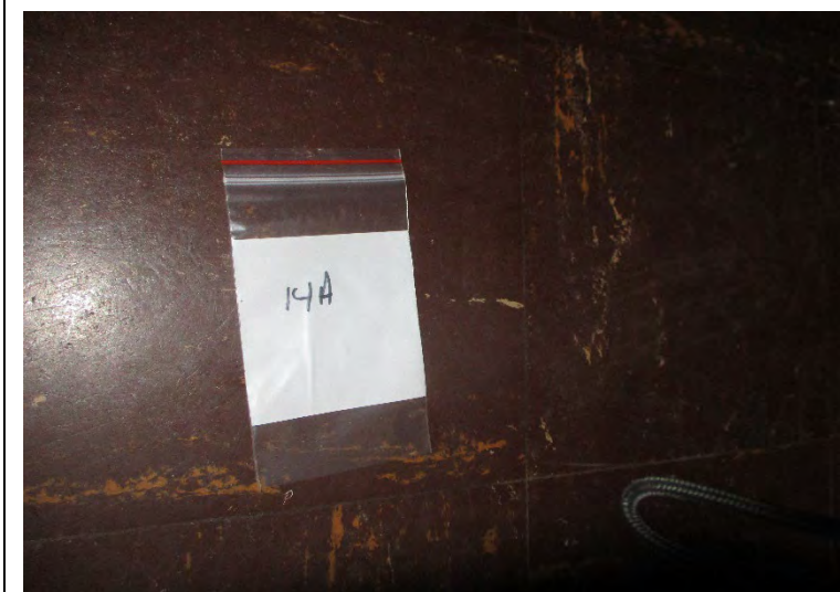
Photo 15. A view of asbestos-containing 9"x9" floor tile in the Kitchen closet in the 5970 Audubon building
