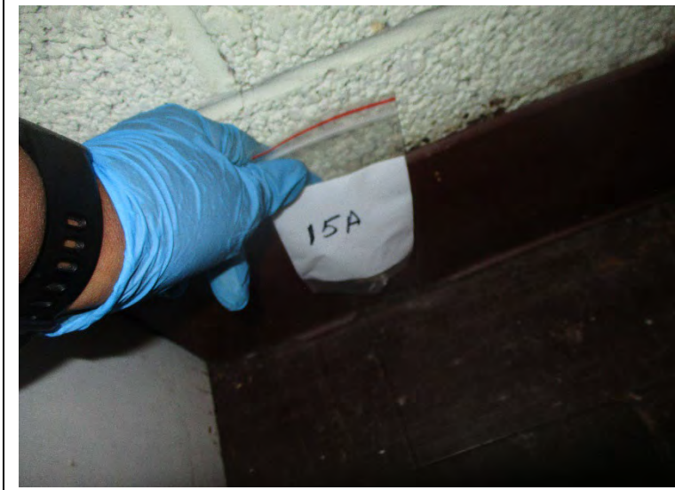
Photo 16. A view of asbestos-containing cove-base in the kitchen closet in the 5970 Audubon building
