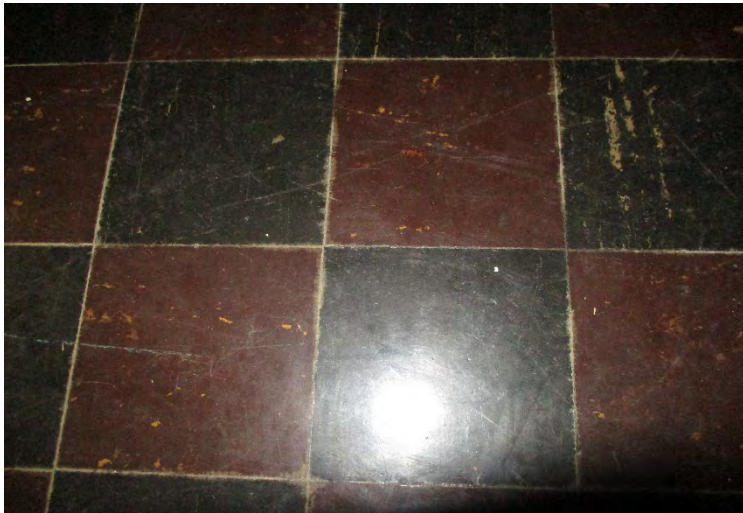
Photo 20. A view of asbestos-containing 9"x9" floor tile in the hallway
