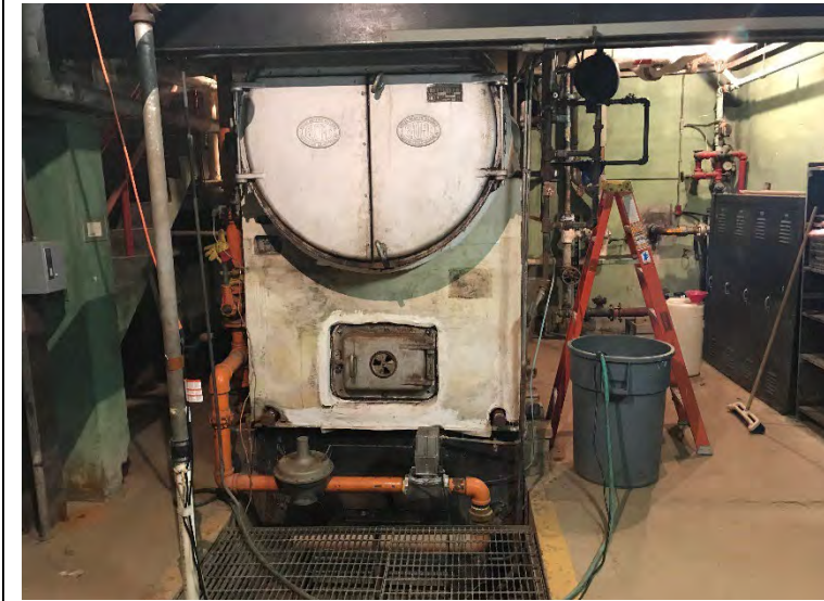
Photo 13. Audubon basement furnace
