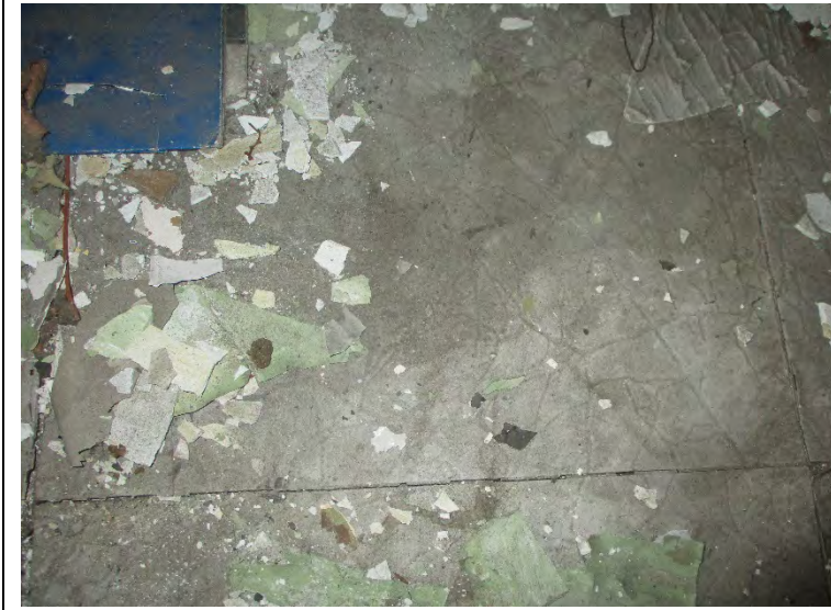
Photo 7. View of asbestos-containing 12" x12" White floor tile in the northwest bedroom of 2253 Sheridan
