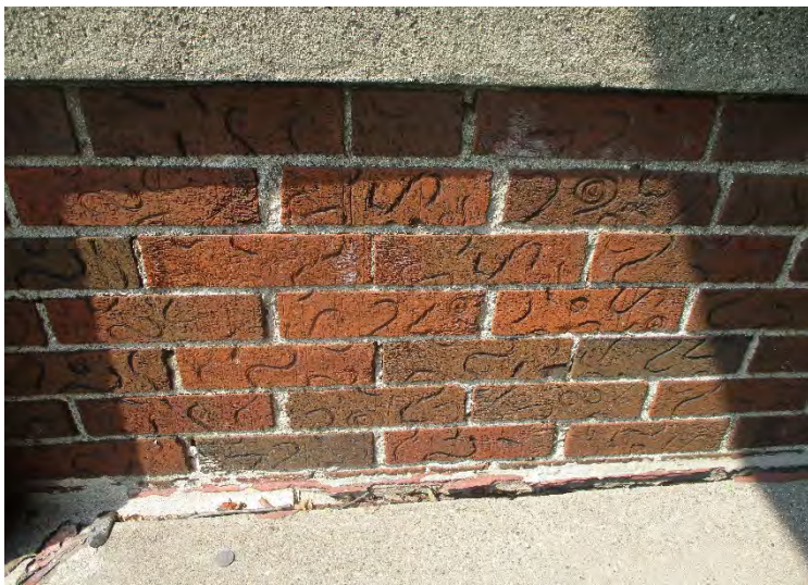
Photo 6. View of asbestos-containing red porch caulk
