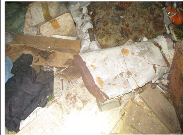
Photo 5. View of Asbestos-containing duct wrap on the ground
