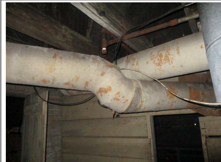
Photo 5. View of asbestos-containing duct insulation
