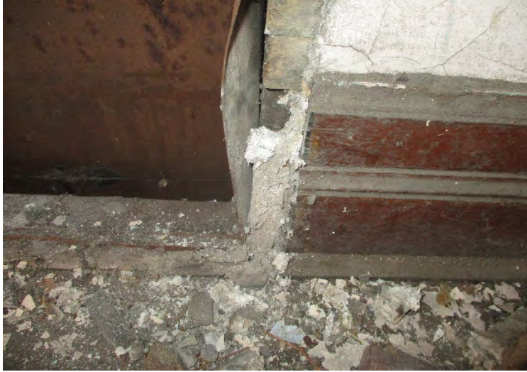
Photo 4. View of asbestos-containing duct insulation
