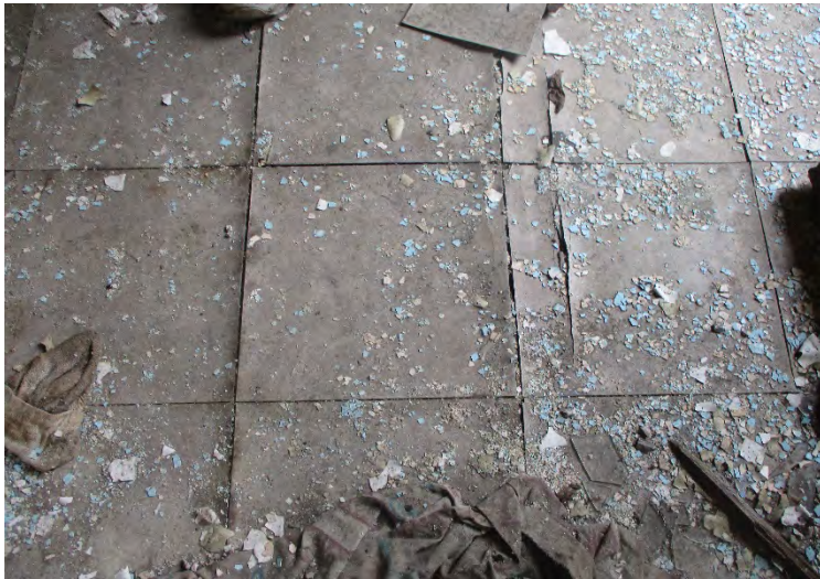
Photo 5. View of asbestos-containing floor tile
