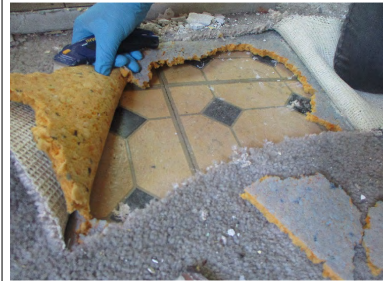
Photo 4. View of black and white 12" x12" floor tile with asbestos-containing Cream floor tile beneath in the southwest bedroom of 2251 Sheridan
