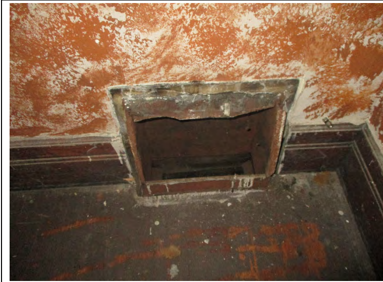
Photo 5. View of asbestos-containing duct paper insulation
