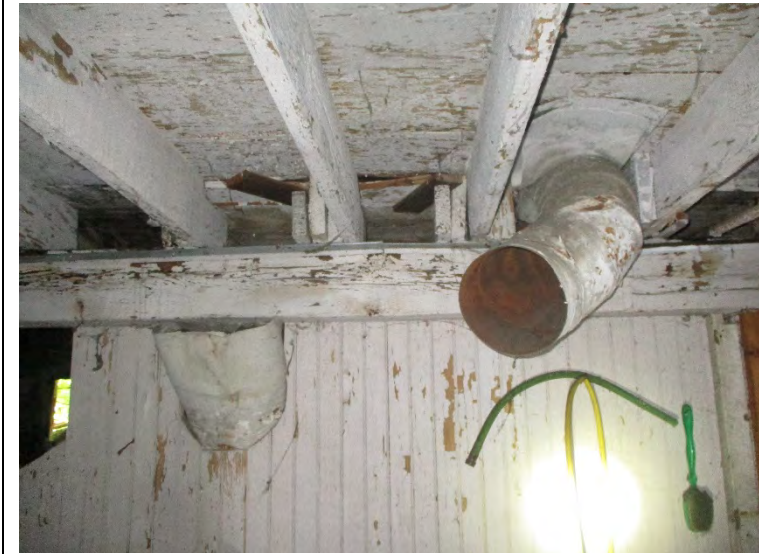
Photo 4. View of Asbestos-containing duct wrap
