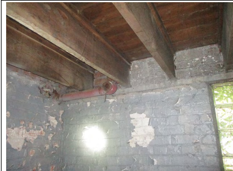
Photo 6. View of asbestos-containing pipe joint insulation
