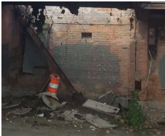
Buckling and loose masonry - first floor
