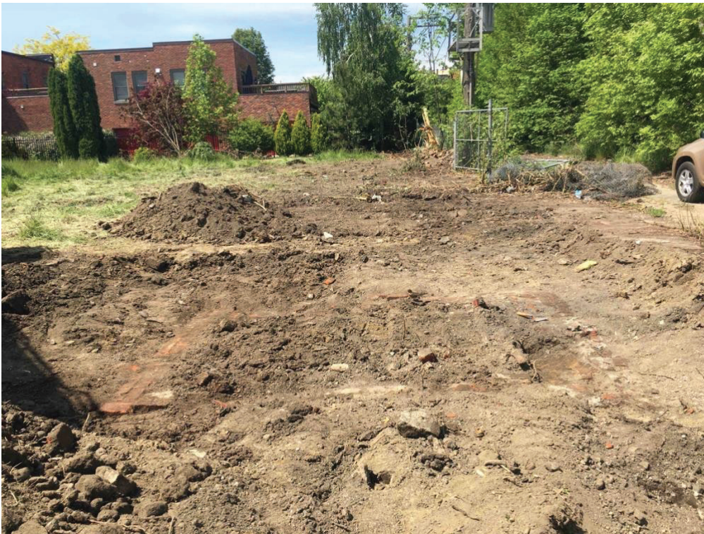
Feature 1 of 20WN12217 (stable foundation), facing west; trench has not been excavated to the west of it yet (May 19, 2021).
