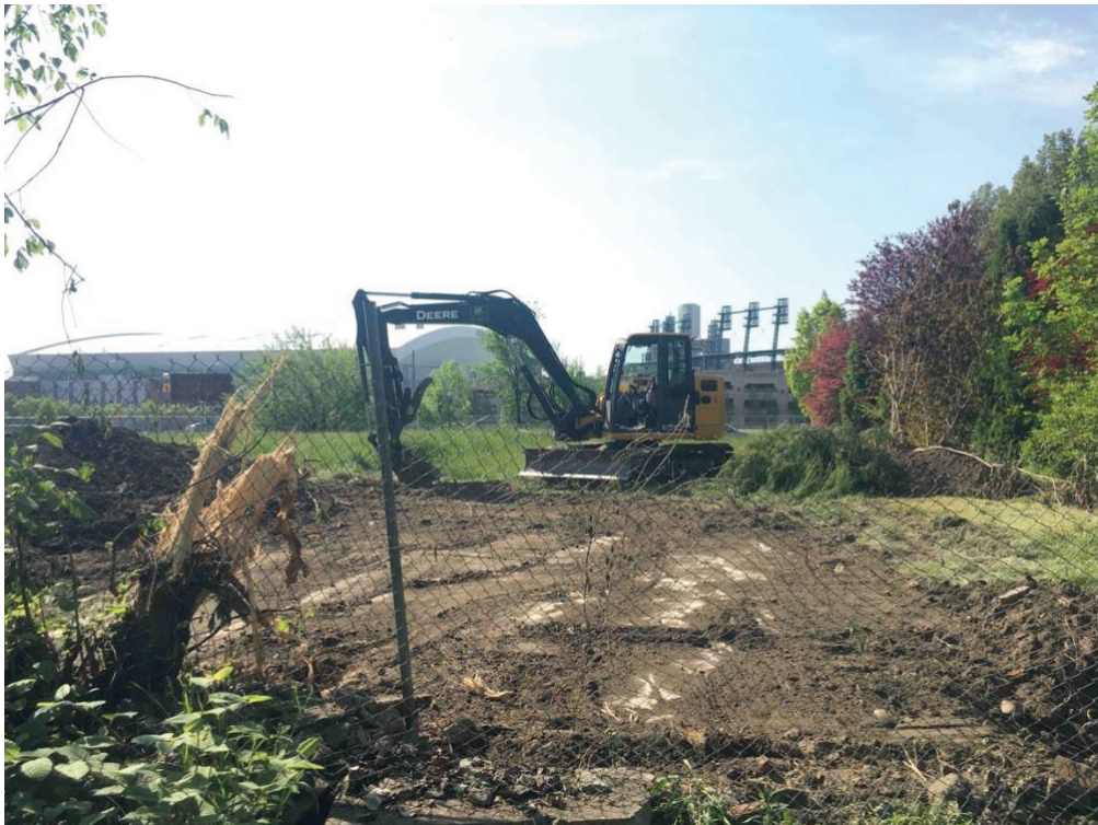
Feature 2, 20WN1227, with the concrete slab foundation is fully exposed. Facing south from alley through the fence (May 20, 2021).
