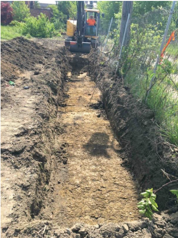
Central portion of the trench; the excavator has stopped on the east side of Feature 1 of 20WN12217 (stable foundation) (May 18, 2021).
