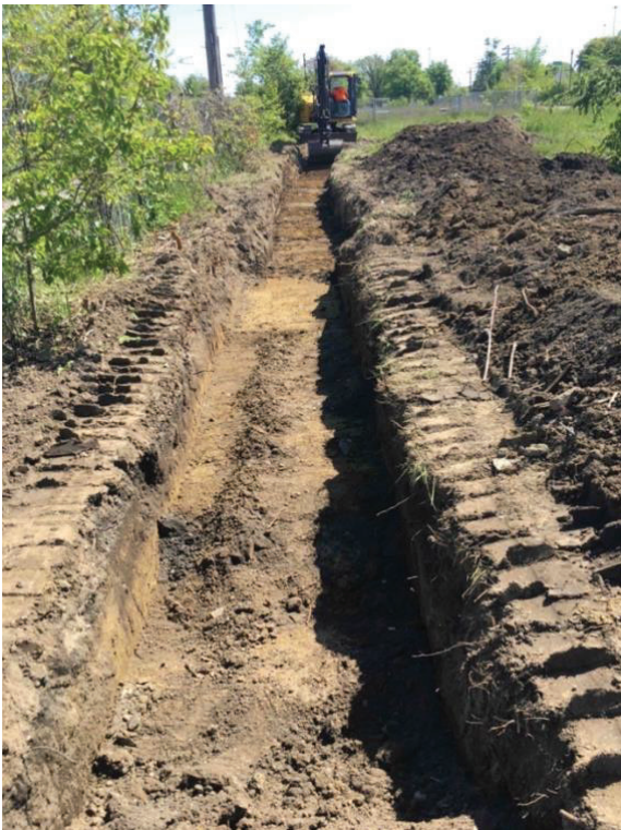
Facing west from east end of trench along the portion of the trench that was excavated on May 17, 2021 (approximately the east half of the trench; photo taken May 18, 2021).
