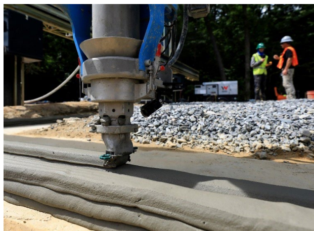
The printer head of a giant 3D printer begins laying cement for the foundation of a Habitat for Humanity home. Consociate Media
