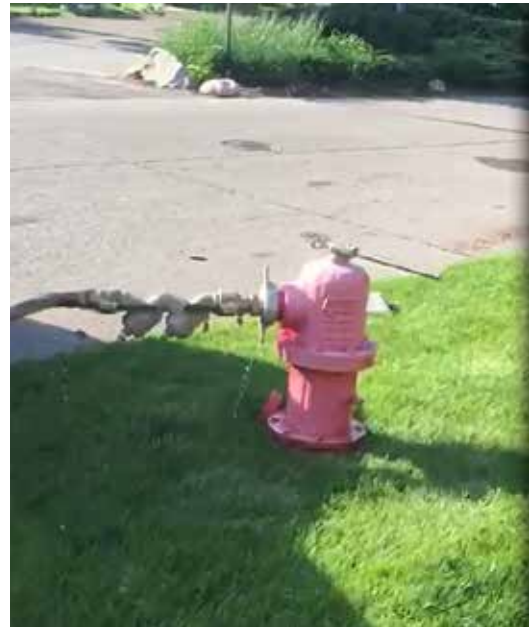
Unauthorized fire hydrant usage
