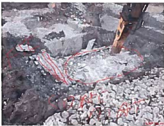
Pictures of some of the unexpected underground obstructions
