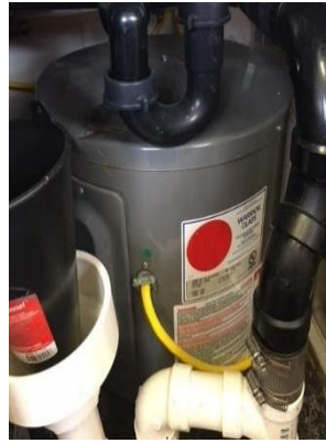
Tank water heater
