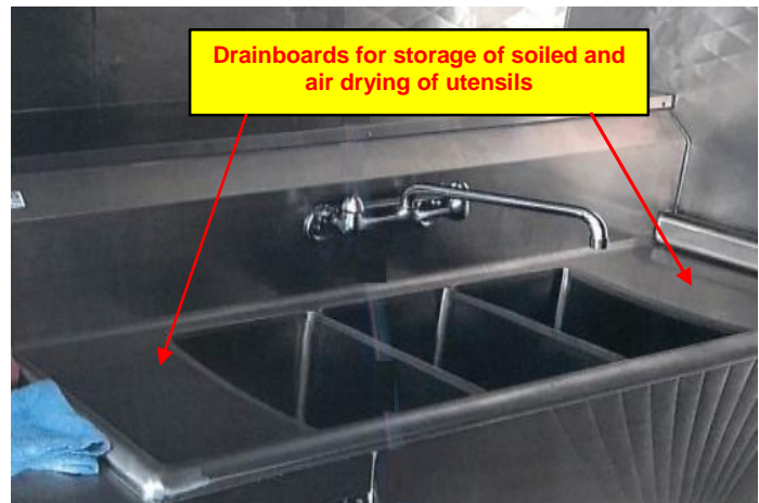
Fixed 3-compartment set up with drainboards
