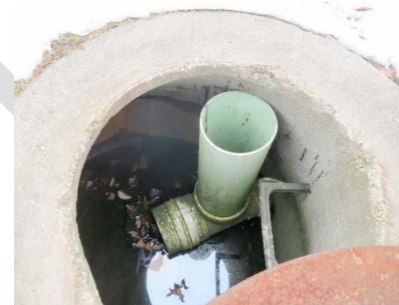
Figure 10-26 Upturned underdrain with a capped tee connection
