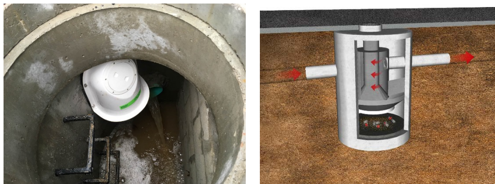
Figure 5-9 Gross Solids Removal Devices
