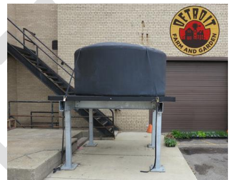
Detroit Farm and Garden cistern
