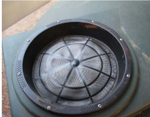
Figure 10-5 Filter at the Inlet on a Cistern
