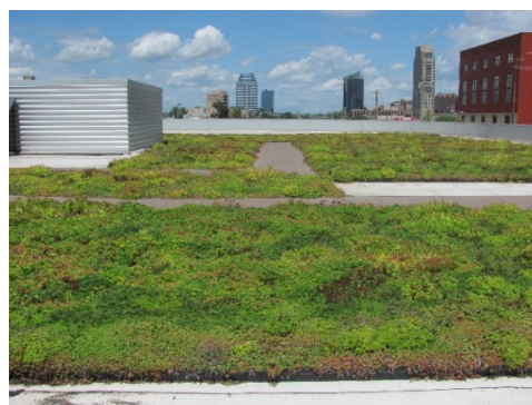
Figure 12-4 Extensive living roof
