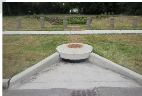
Figure 8-19 Curb cut bypassing CB
