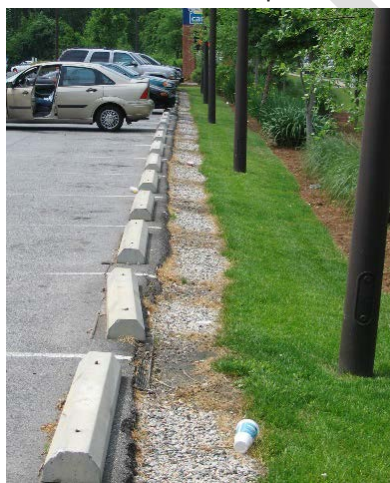
Figure 8-24 Vegetated filter strip leading to bioretention
