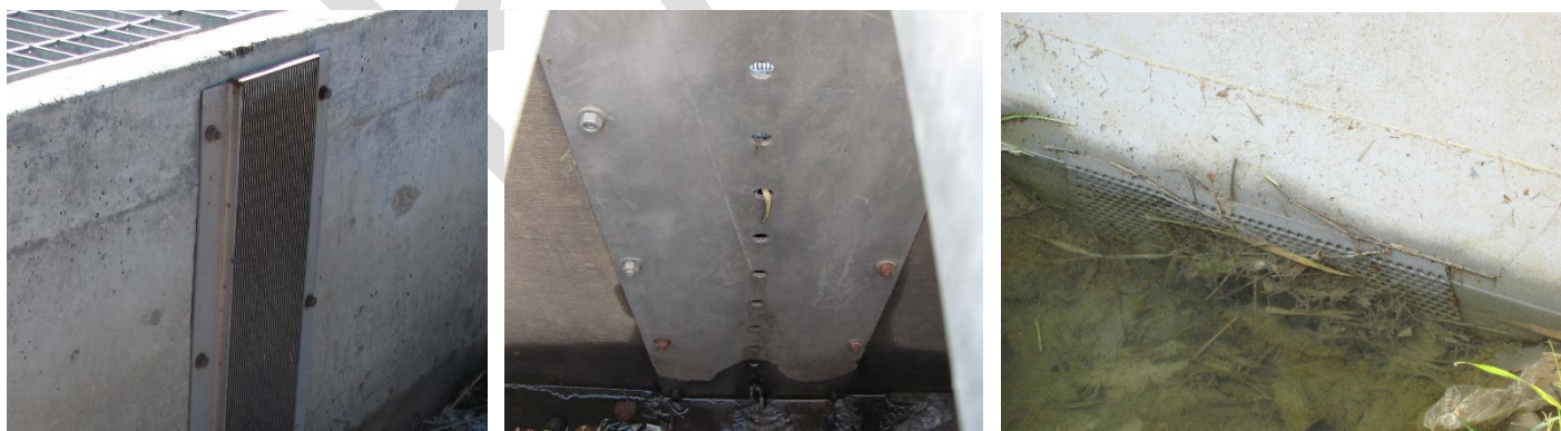
Specialty screen protecting orifice plate from clogging, outside (left); orifice plate, inside (center); clogged poorly designed screen (right)
