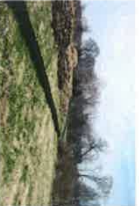
Silt fence installed at construction site Source: U.S. EPA, 2008, NPDES, Construction Site Stormwater Runoff Control
