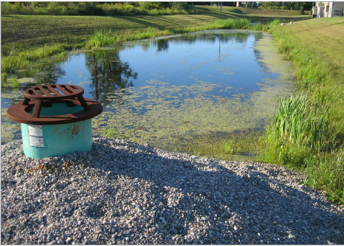
Retention basin with outlet riser in the foreground of the photo
