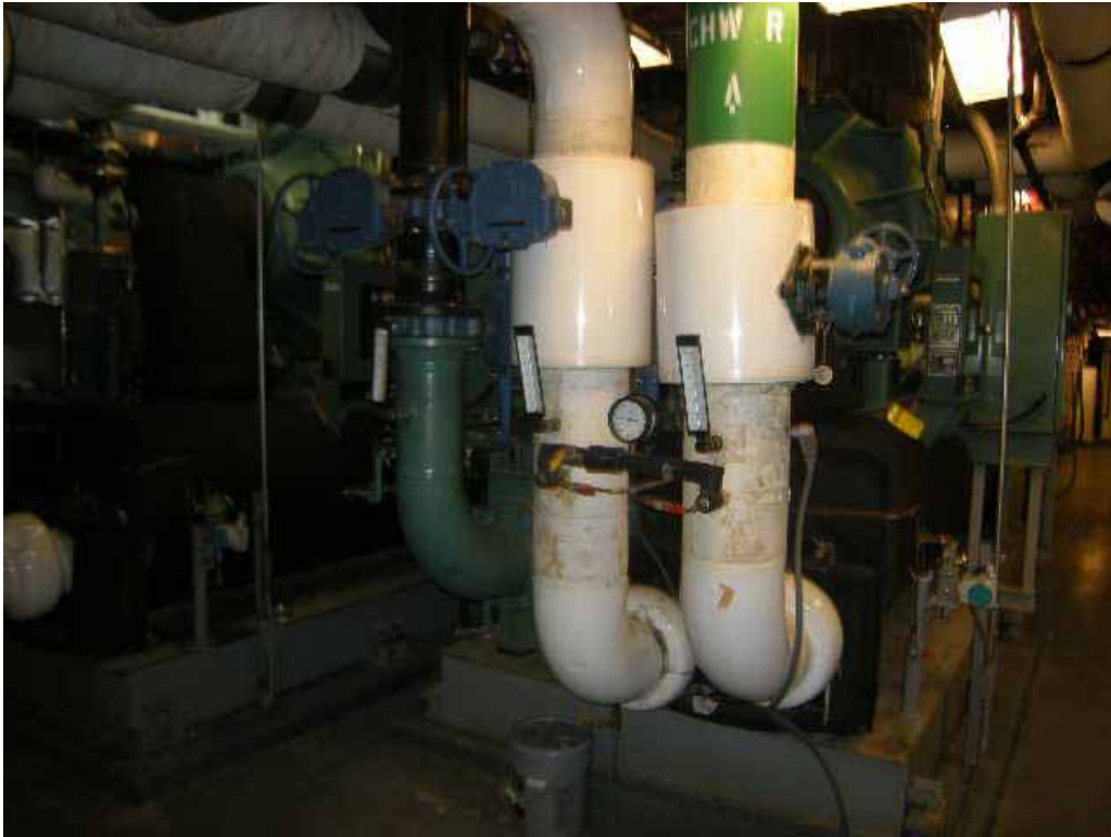
Detroit Institute of Arts HVAC Equipment
