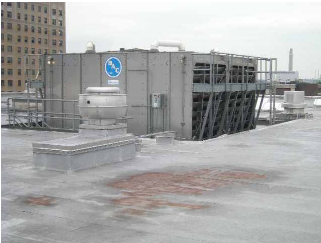
Detroit Institute of Arts Roof Area & HVAC Equipment
