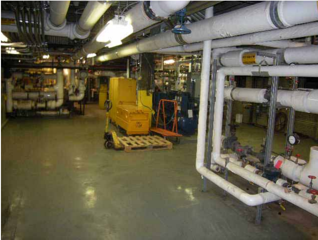
Detroit Institute of Arts HVAC Equipment
