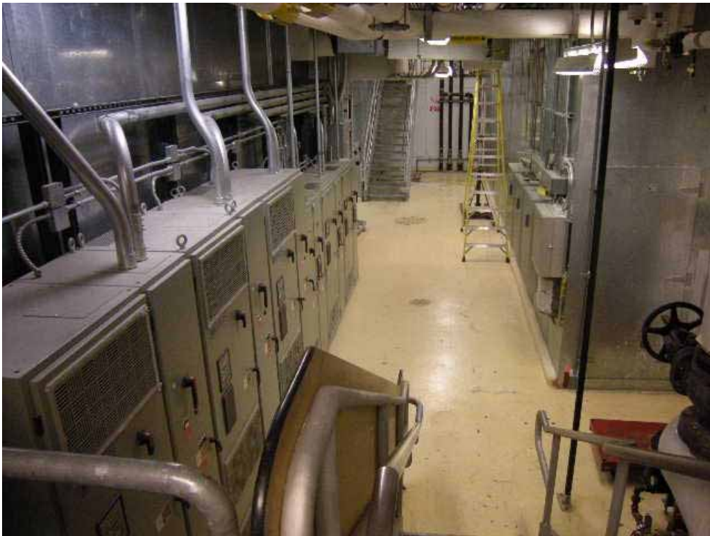
Detroit Institute of Arts HVAC Equipment
