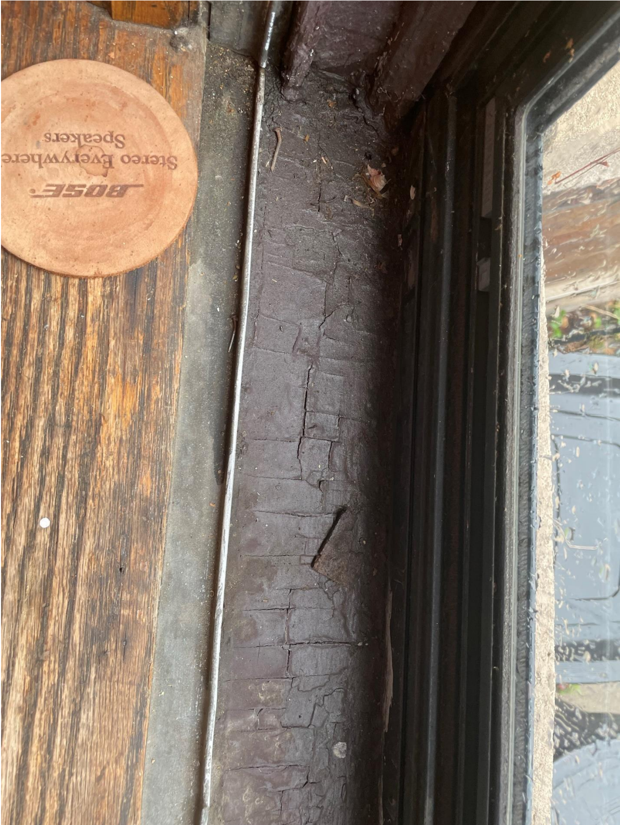
Window #4 – water damage
