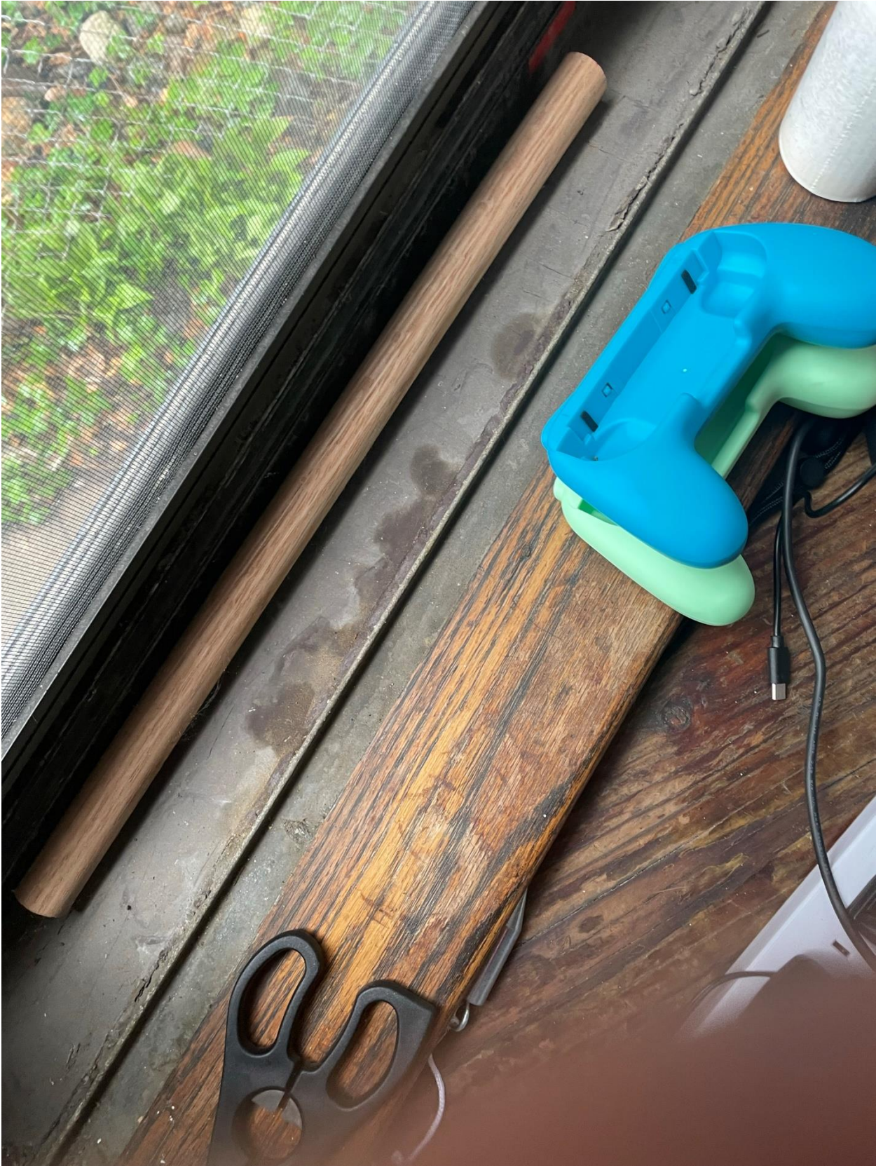
Window #5 – Water Damage
