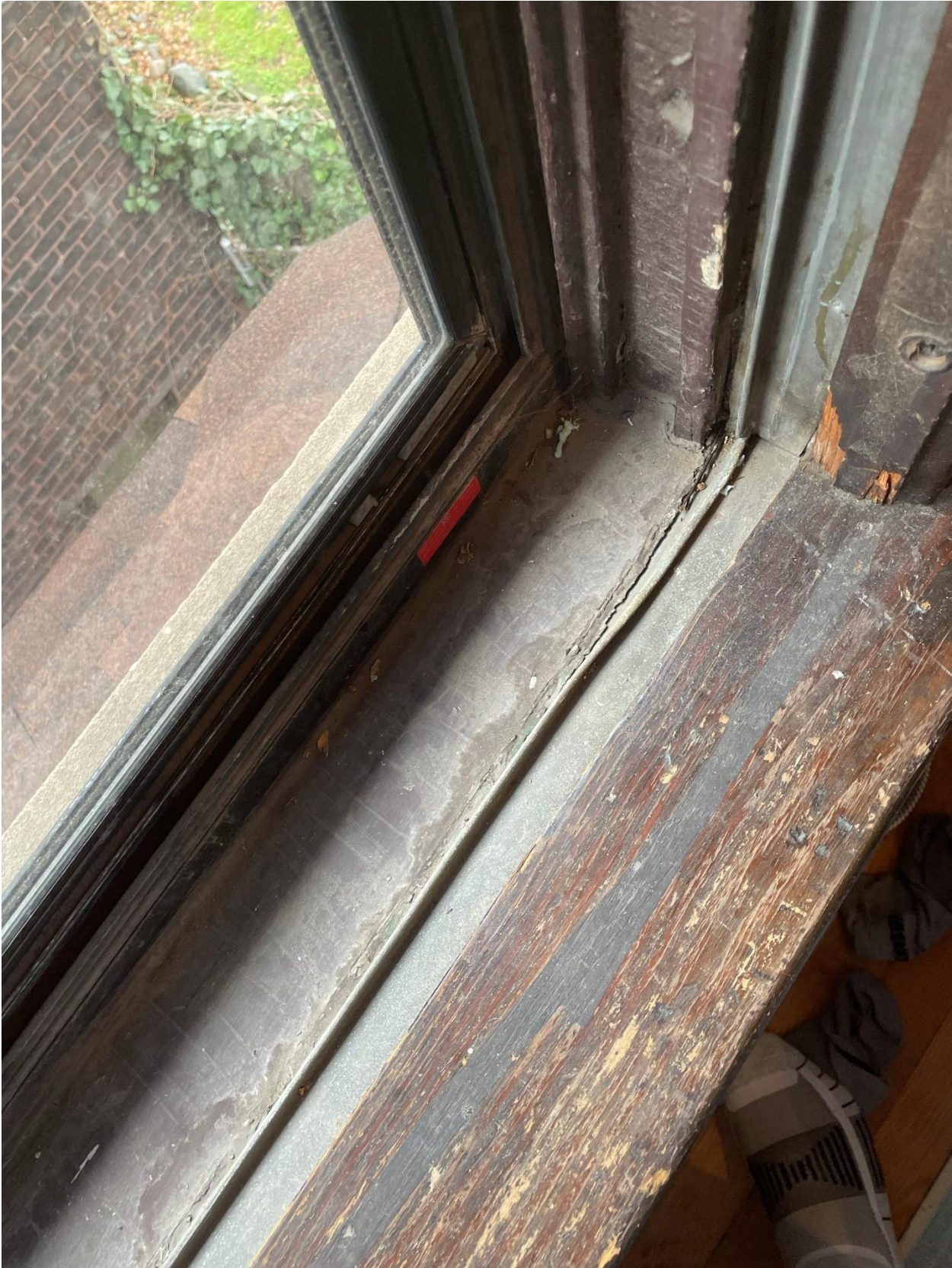
Window #13 – Water Damage
