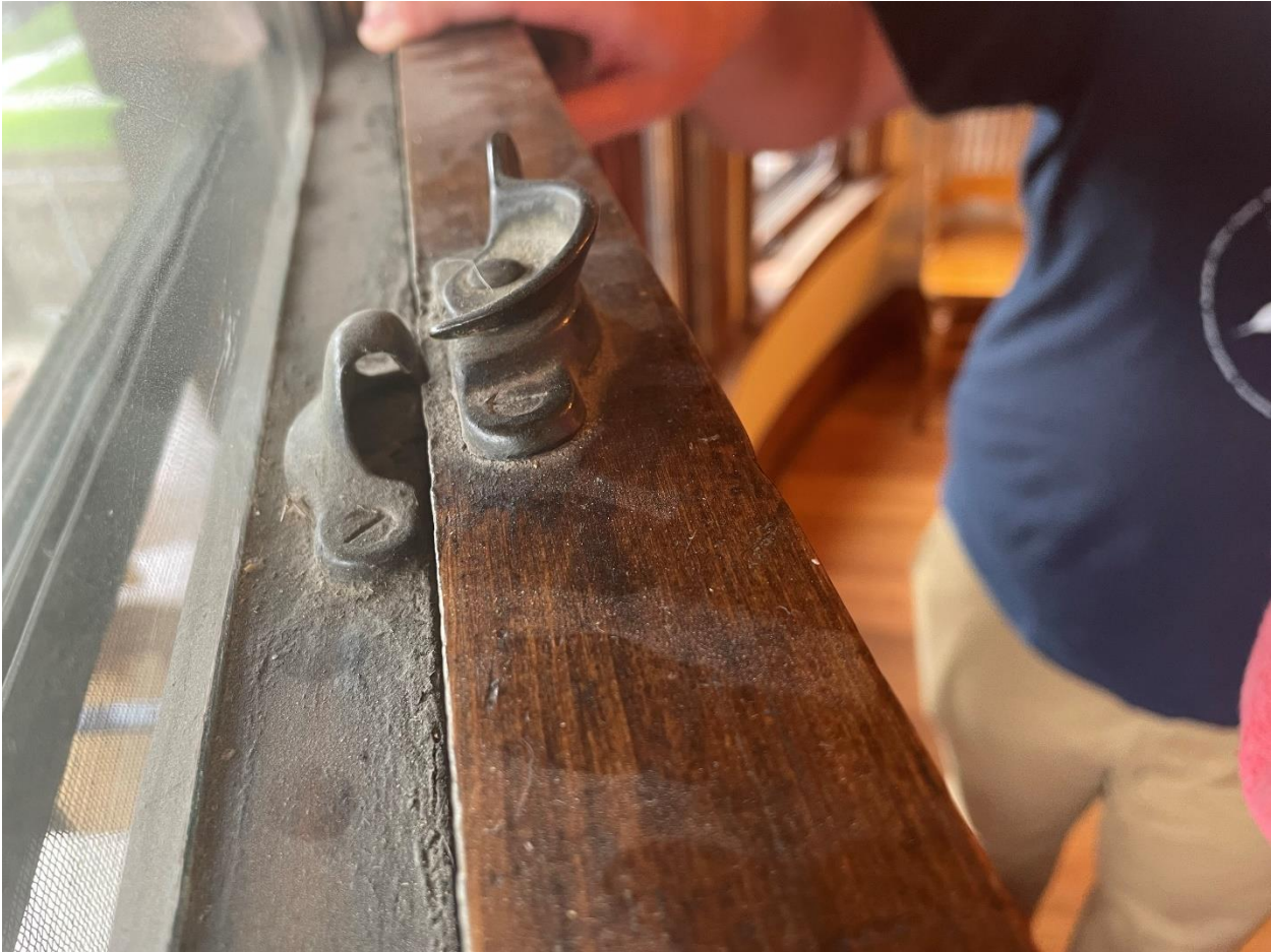
Window #2 – Uneven panes that cannot lock.
