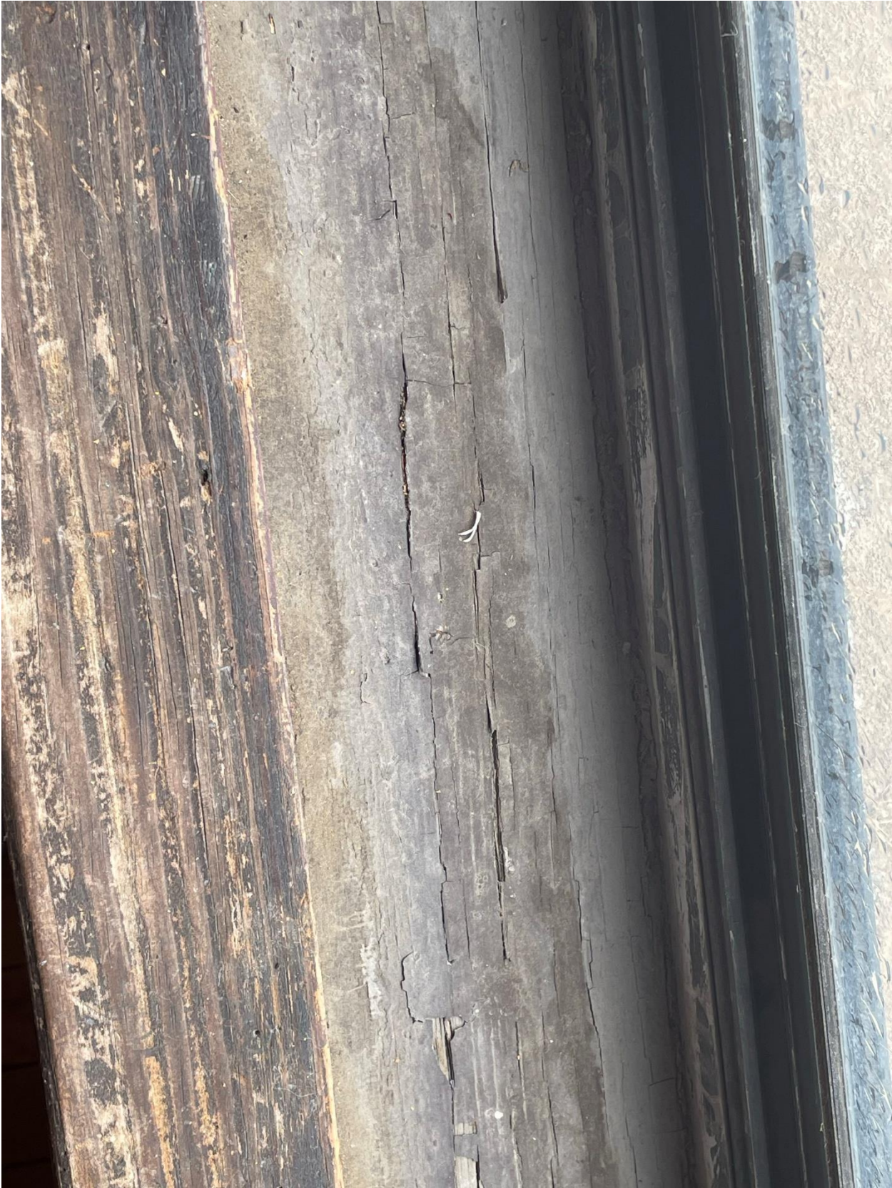
Window #11 – Water Damage
