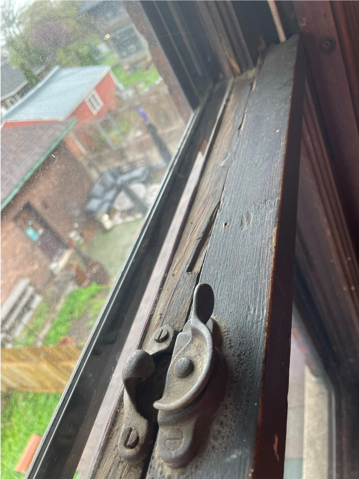
Window #15 – Panes are different sizes so cannot be closed
