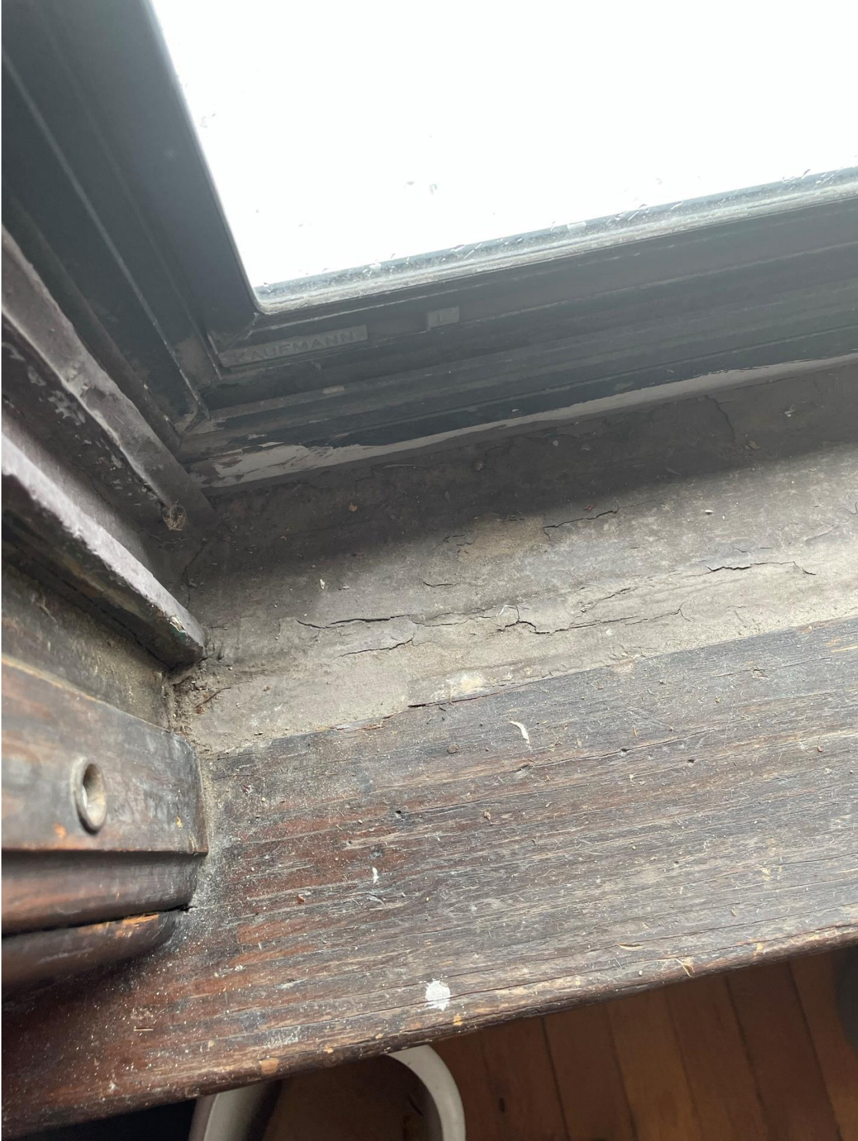
Window #9 – Water Damage
