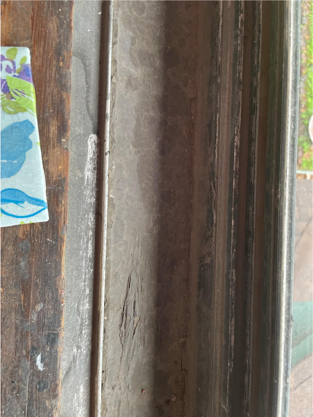
Window #15 – Water Damage
