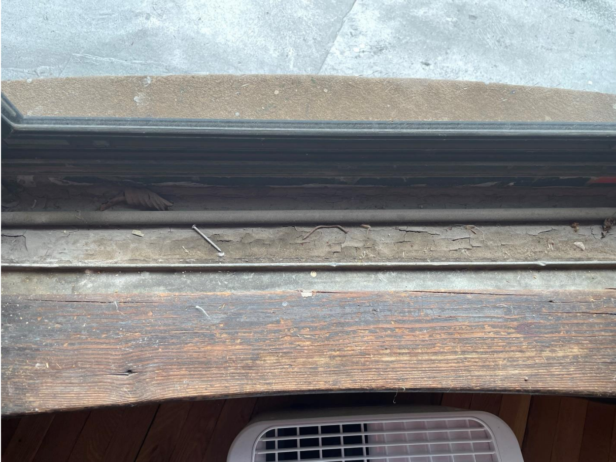
Window #10 – Water Damage
