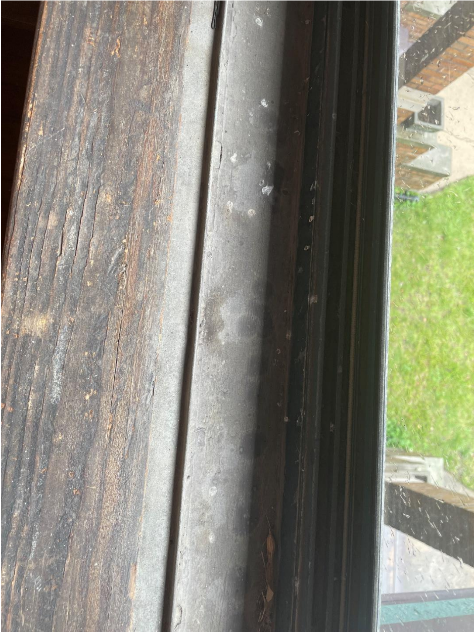
Window #8 – Water Damage
