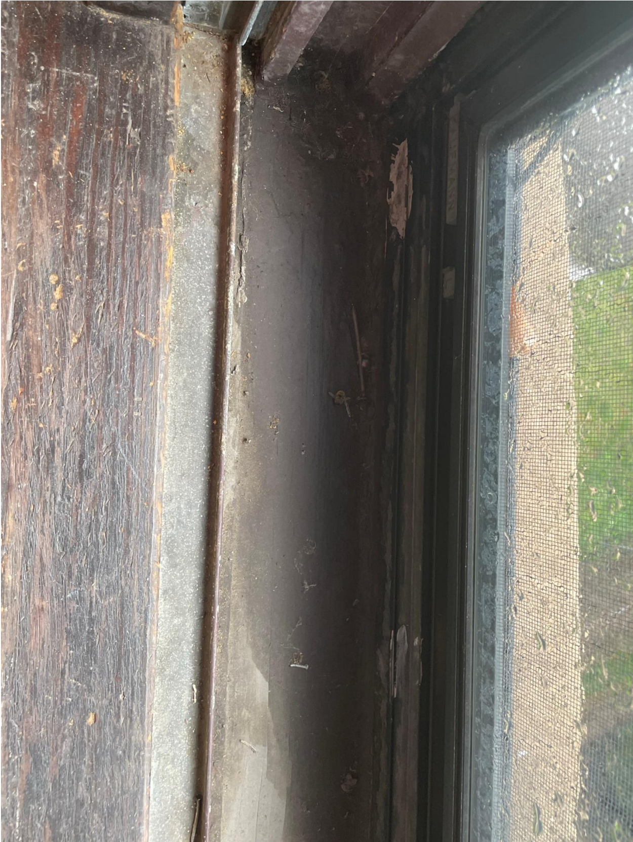
Window #12 – Water Damage
