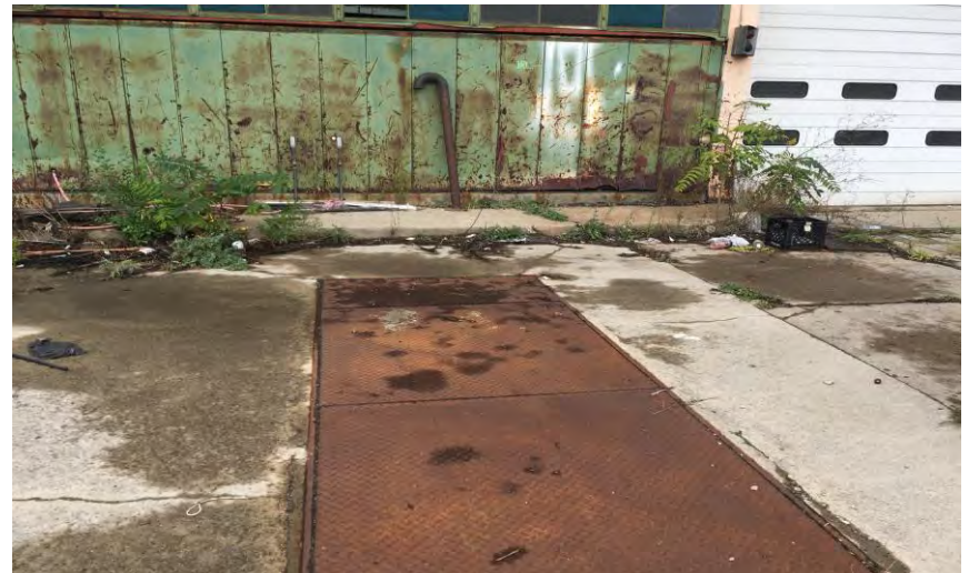
Unable to remove and determine what is under the plates. Located on the East Side of the Bus Garage
