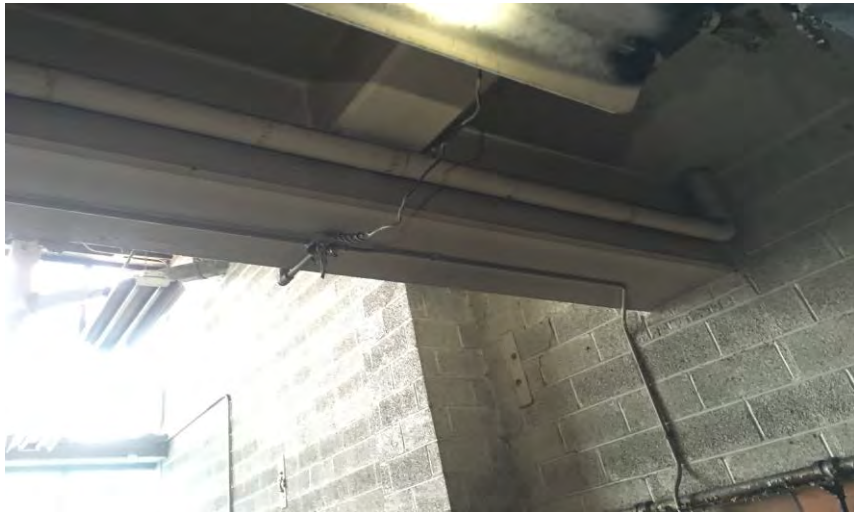
Assumed Aircell pipe insulation in Room BB1121 in Bus Garage.
