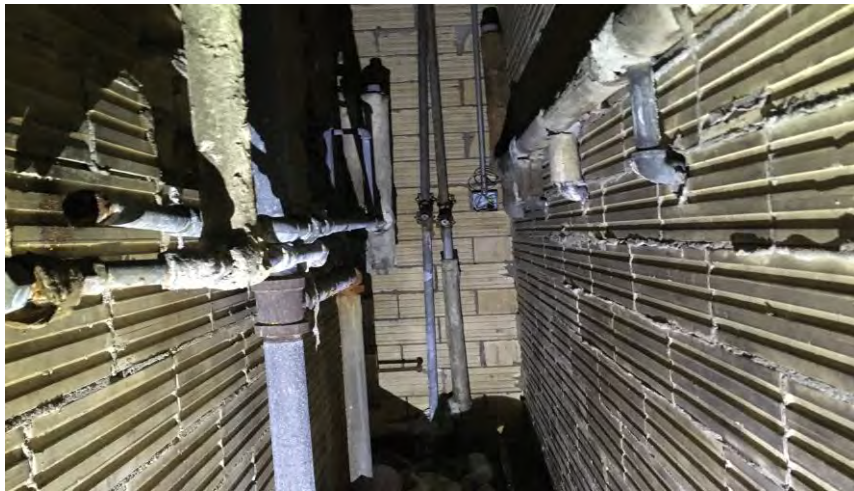
Mud Joints on the Non-asbestos Paper Insulation in the Men's Bathroom Plumbing Closets in the Bus Garage Sample #10
