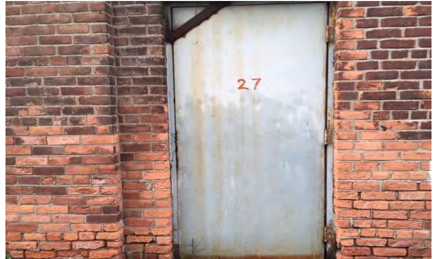
Exterior Door and Window Caulk on Carriage Storage Building Sample # 34
