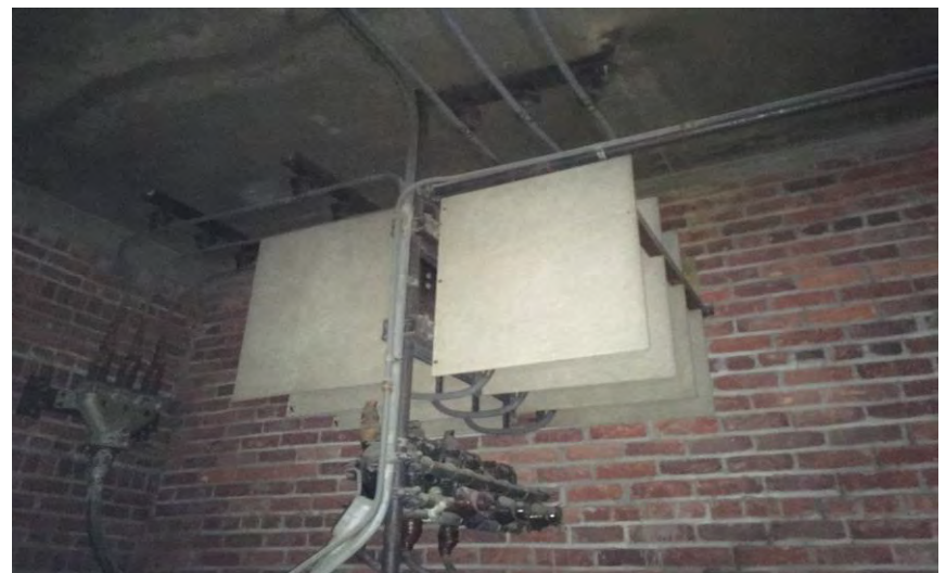
Transite Panels in the Boiler Building Electrical Room
