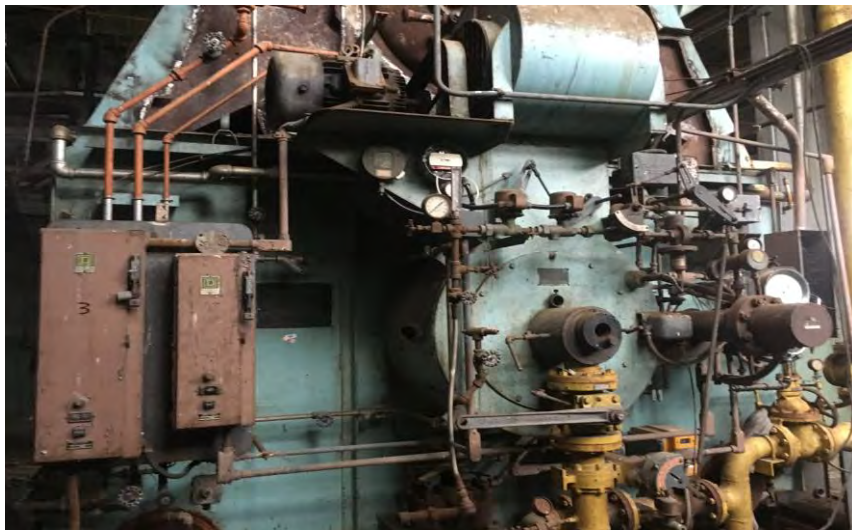
Mercury Containing Switches on the Boiler in the Boiler Building
