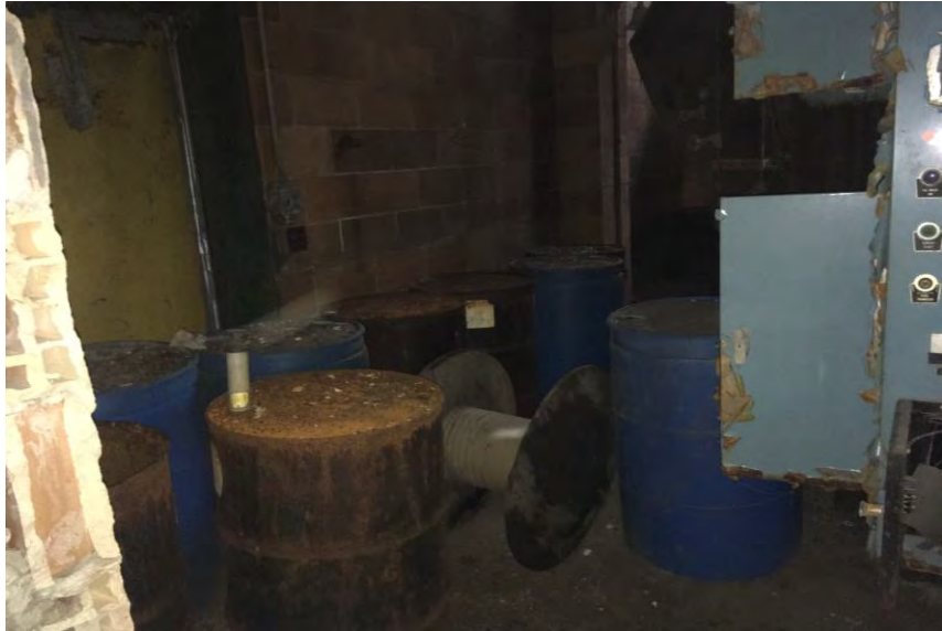
Drums in the Boiler Building
