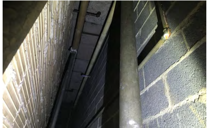
Asbestos Block Pipe Insulation Sample #11 in the Bathroom Plumbing Closets in the Bus Garage
