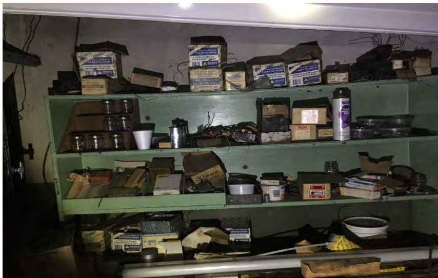
Florescent Bulbs and Ballasts in the Basement Electrical Room in the Terminal Building
