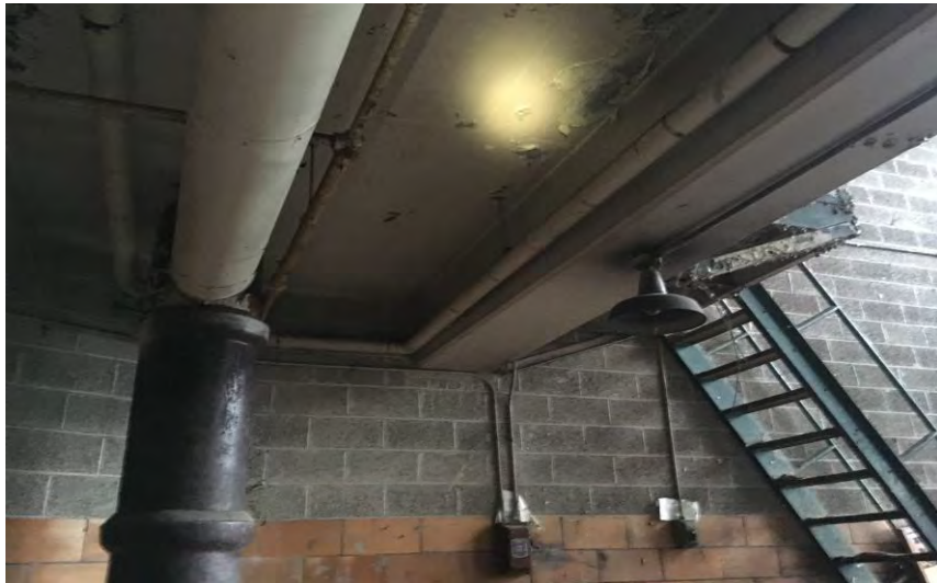
More Assumed Aircell pipe insulation in Room BB1121 in Bus Garage.
