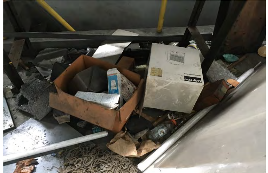
Mercury Vapor Bulbs and Ballasts in the Electrical Room above Room BB1108 in the Bus Garage
