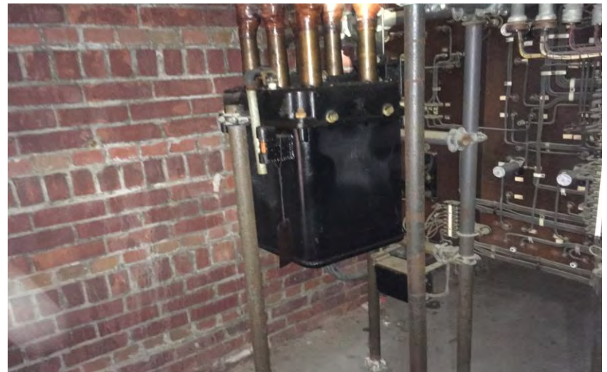
Oil Filled Transformers possible PCB Oil and Stained Concrete in the Electrical Room in the Boiler Building
