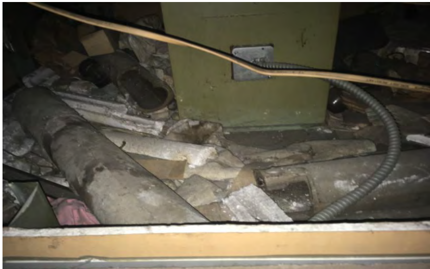
Pipe Insulation that is above the Message Boards in the Terminal Building
