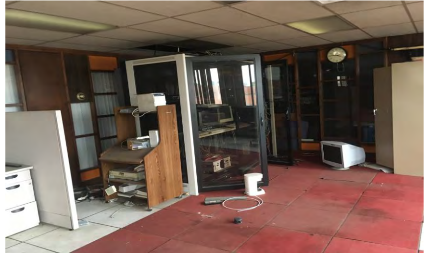
Monitors, UPS, Mercury Switch Thermostat and Computers on the 2 nd Floor of the Terminal Building
