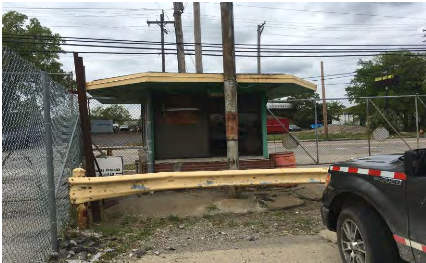
Caulk Around Windows in the Guard Shack Sample 4a
