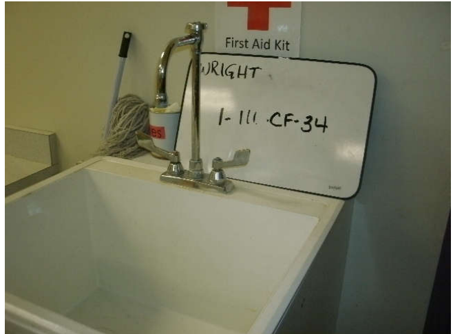
Photo 34: Classroom faucet, located on the 1st floor, in room 111.
