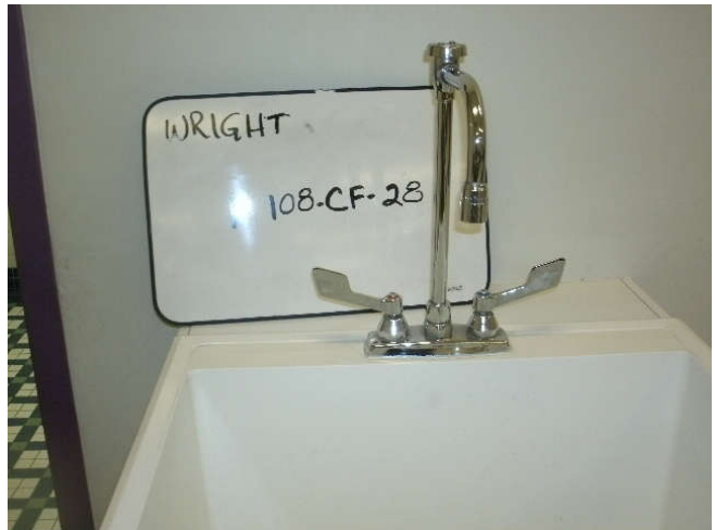
Photo 28: Classroom faucet, located on the 1st floor, in room 108.
