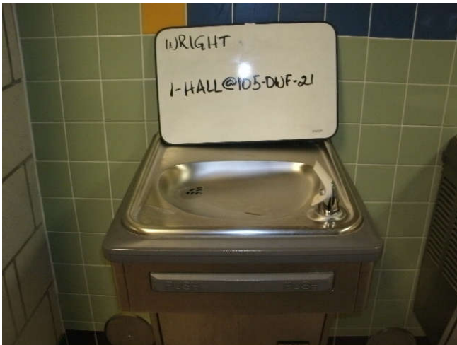
Photo 21: Drinking water fountain, located in a 1st floor hallway, to the right of room 105 – left fixture.
