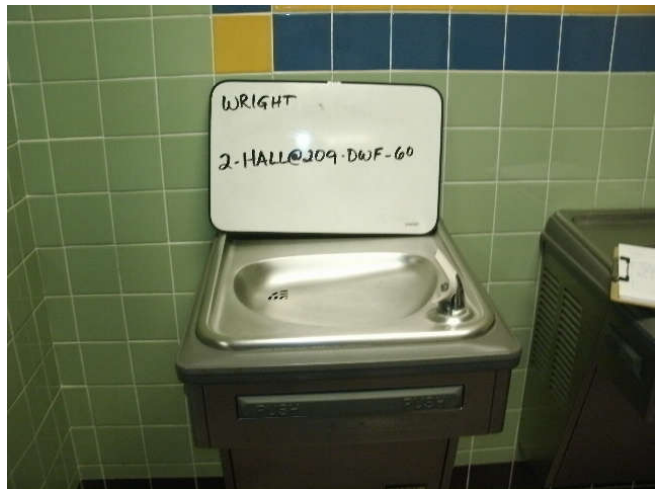
Photo 60: Drinking water fountain, located in a 2nd floor hallway, near room 209 - left fixture.
