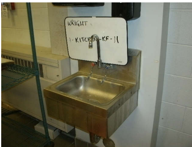
Photo 11: Kitchen faucet, located on the 1st floor in the kitchen, across from KF-10 (hand washing).
