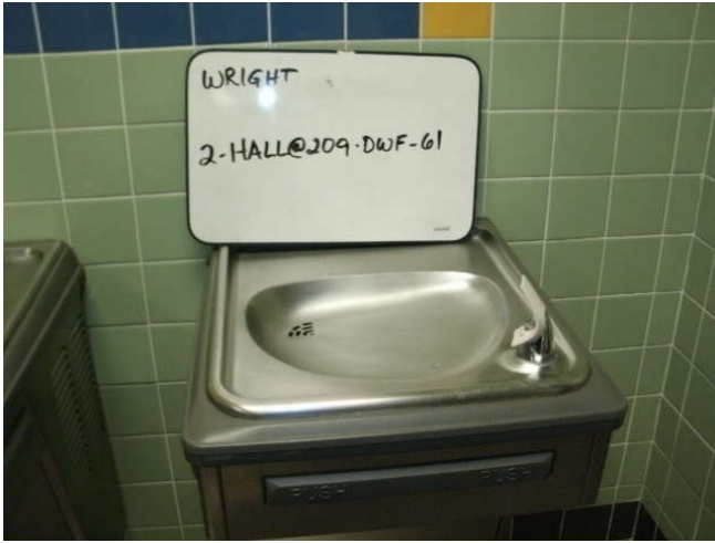
Photo 61: Drinking water fountain, located in a 2nd floor hallway, near room 209 - right fixture.
