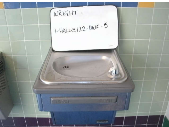
Photo 5: Drinking water fountain, located in a 1st floor hall, across from room 122 – right fixture.
