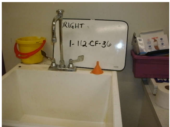
Photo 36: Classroom faucet, located on the 1st floor, in room 112.
