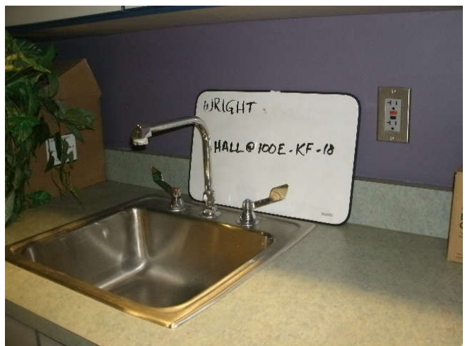
Photo 18: Kitchen faucet, located in a 1 st floor hall in the main office area, across from room 100E.
