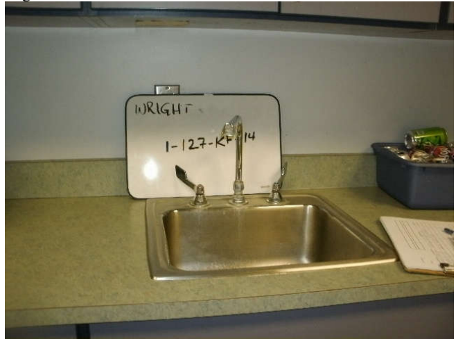
Photo 14: Kitchen faucet, located on the 1 st floor, in room 127 (teacher's lounge).
