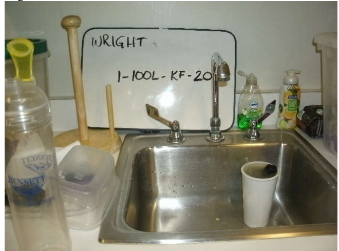
Photo 20: Kitchen faucet, located on the 1st floor, in room 100L, in the main office area.
