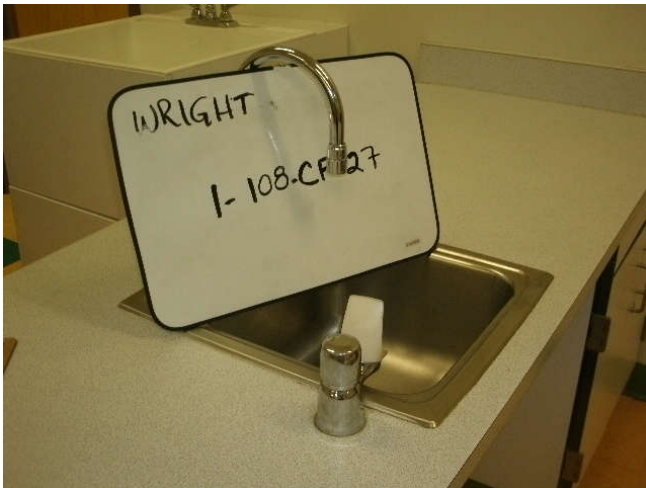
Photo 27: Classroom faucet w/bubbler, located on the 1st floor, in room 108.
