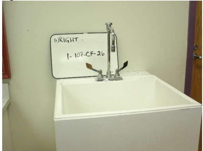
Photo 26: Classroom faucet, located on the 1st floor, in room 107.
