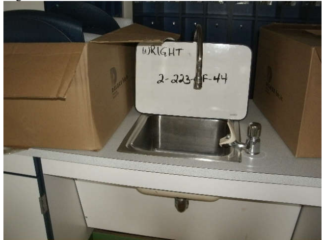
Photo 44: Classroom faucet w/bubbler, located on the 2nd floor, in room 223.
