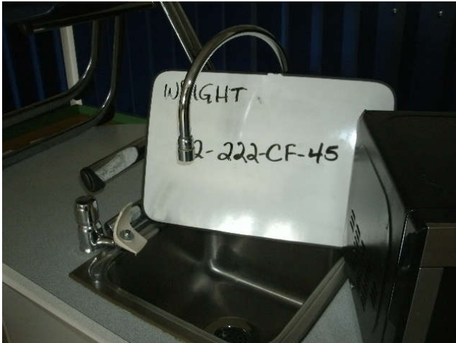
Photo 45: Classroom faucet w/bubbler, located on the 2nd floor, in room 222.
