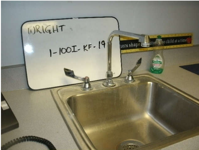
Photo 19: Kitchen faucet, located on the 1st floor, in room 100I, in the main office area.
