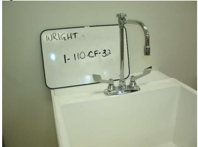
Photo 32: Classroom faucet, located on the 1st floor, in room 110.
