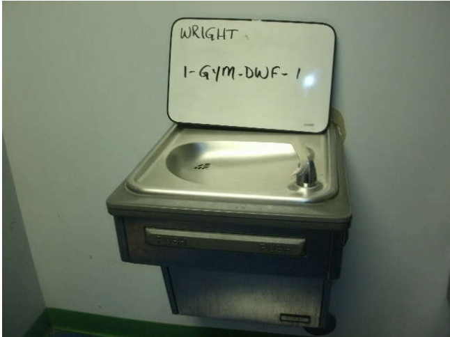
Photo 1: Drinking water fountain, located on the 1st floor in the gym – left fixture.
