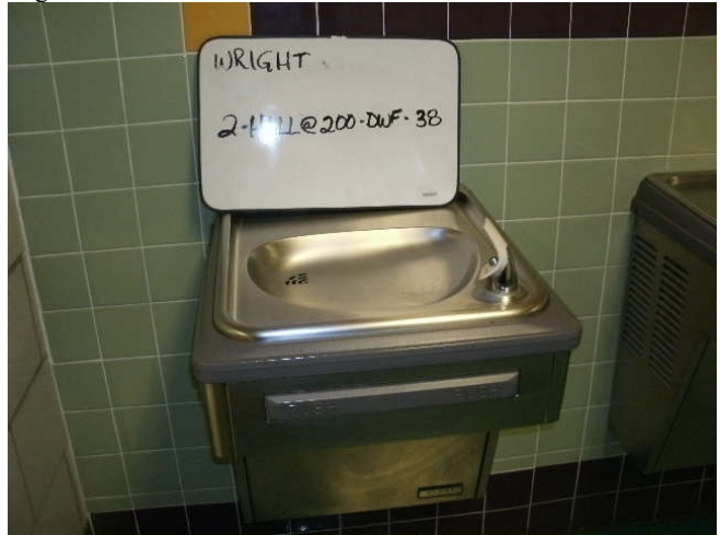
Photo 38: Drinking water fountain, located in a 2nd floor hallway, across from room 200 - left fixture.
