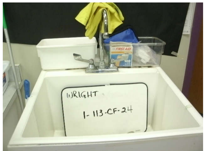
Photo 24: Classroom faucet, located on the 1st floor, in room 113.
