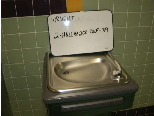
Photo 39: Drinking water fountain, located in a 2nd floor hallway, across from room 200 - right fixture.
