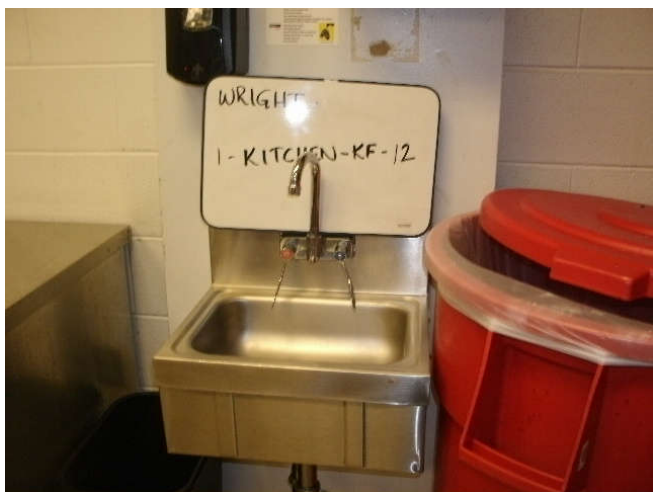
Photo 12: Kitchen faucet, located on the 1st floor in the kitchen serving area (hand washing).
