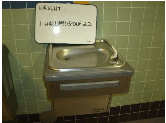
Photo 22: Drinking water fountain, located in a 1st floor hallway, to the right of room 105 – right fixture.
