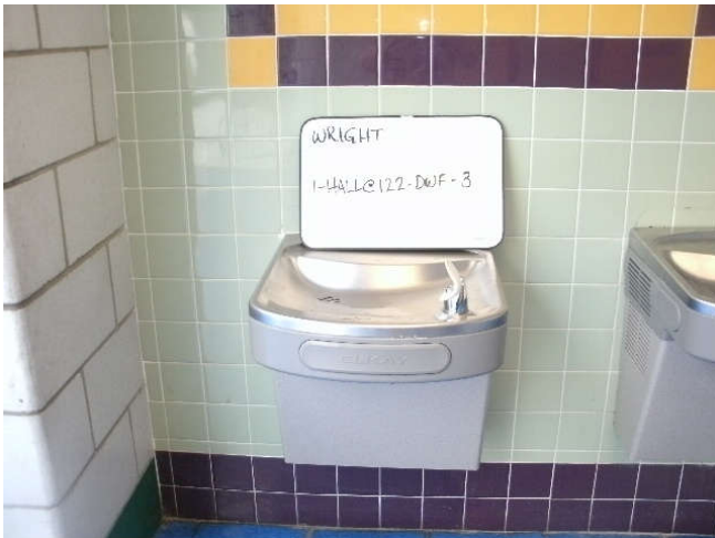
Photo 3: Drinking water fountain, located in a 1st floor hall, across from room 122 – left fixture.
