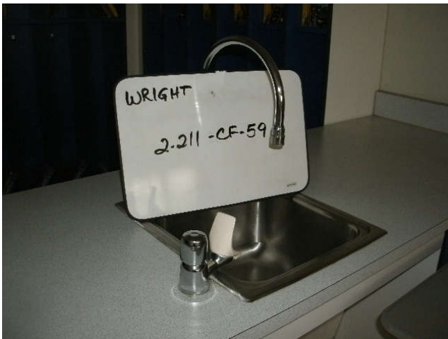
Photo 59: Classroom faucet w/bubbler, located on the 2nd floor, in room 211.
