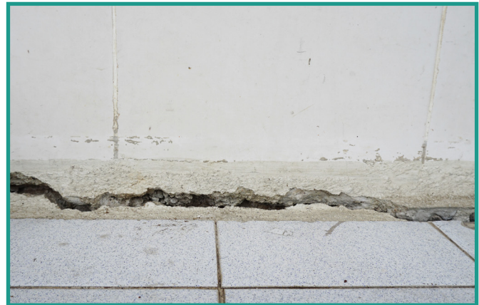
Identify and repair cracks in your basement wall
