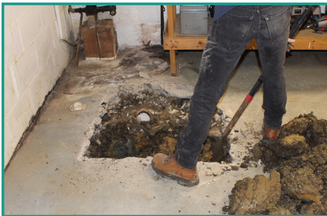
Contractor removing a portion of the basement floor and digging underneath to expose the sewer service line in order to install the backwater valve
