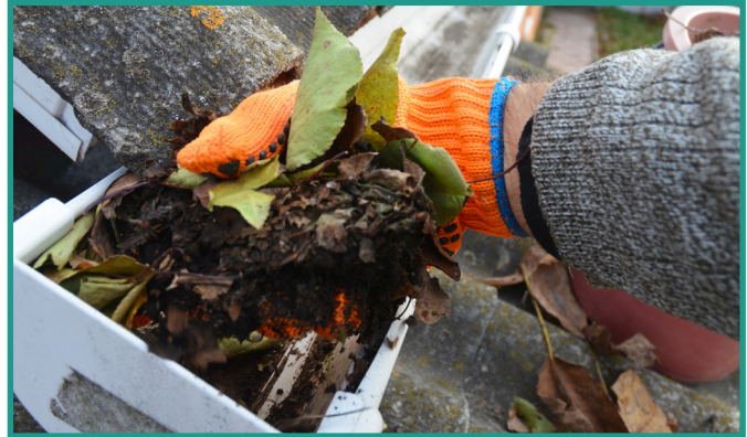
Clean gutters regularly - clogs can lead to rainwater seeping down your wall and into your foundation
