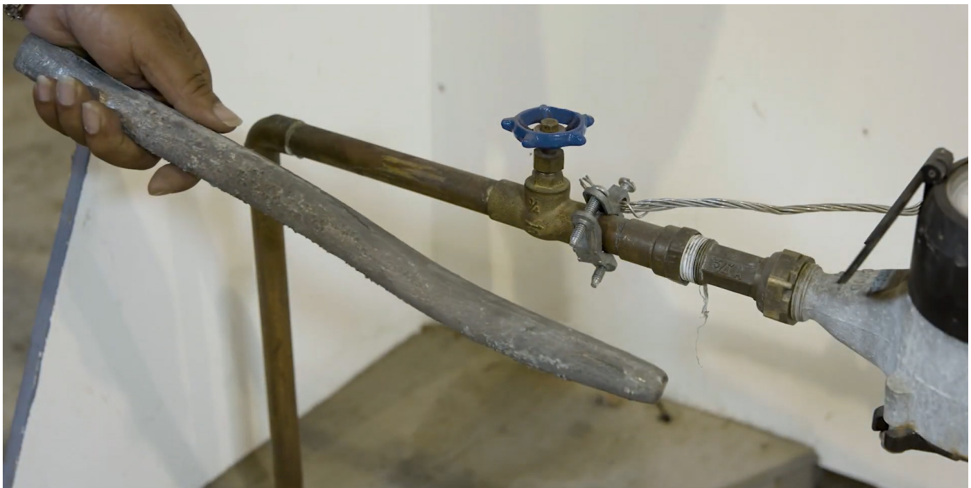
Example of the lead pipe being held up against the copper that has been installed.
