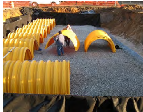
Subsurface Detention Storage
