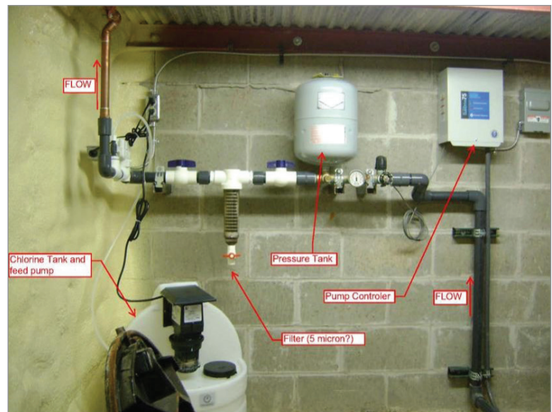
Cedar Street School cistern distribution system, Lansing, MI Photo credit: DC Engineering, PC
