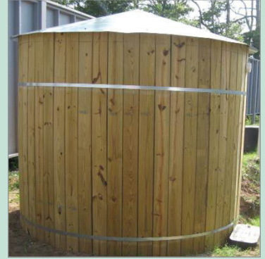
Wood wrapped cistern Pine Knoll Shores, NC
